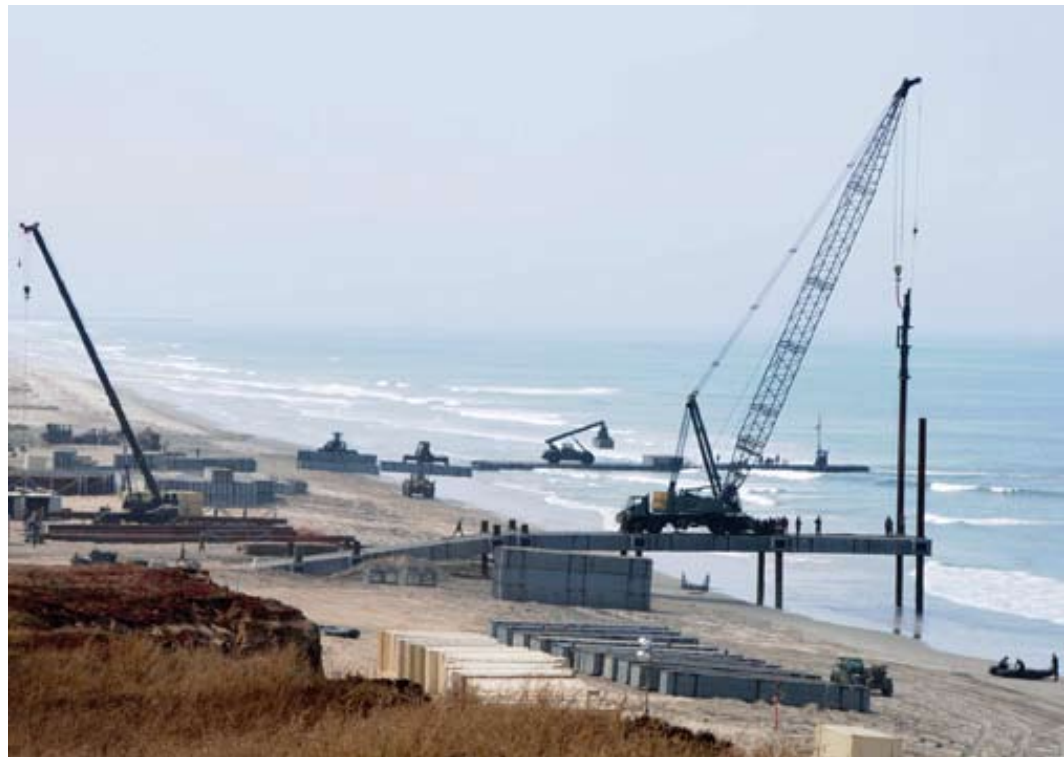
A 175-ton crane moves pile sections into place as the elevated causeway (ELCAS) pier is constructed into the Pacific Ocean. In the distance, a barge ferry is being unloaded on the beach by a Kalmar rough-terrain container handler. Additional pontoon sections for the ELCAS pier are visible in the foreground.
