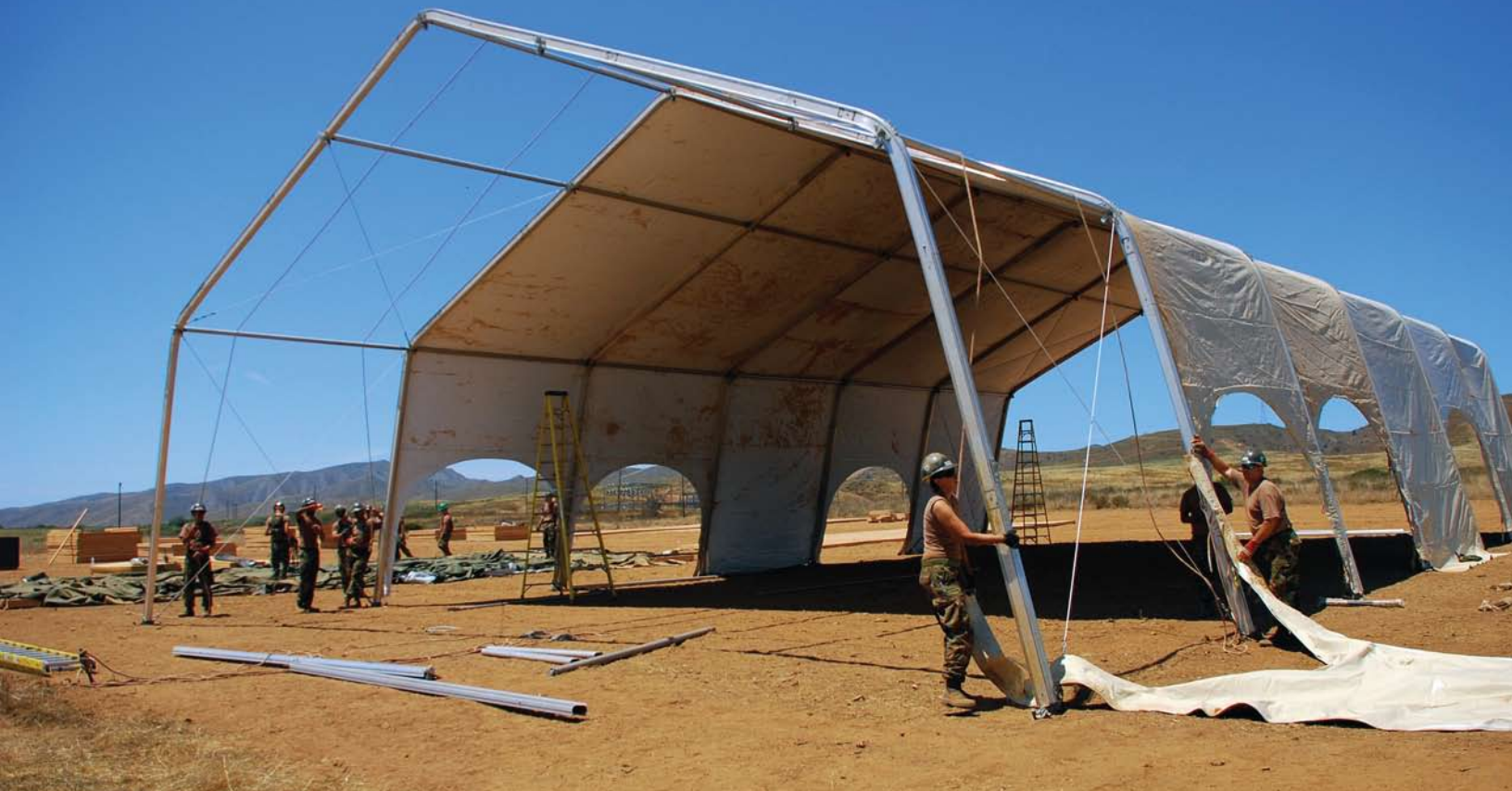
Seabees from Amphibious Construction Battalion 1 erect the metal frame of a tension fabric structure that will be the 700-seat galley (dining facility) for Camp Peguero, the base camp for Pacific Strike 2008.
