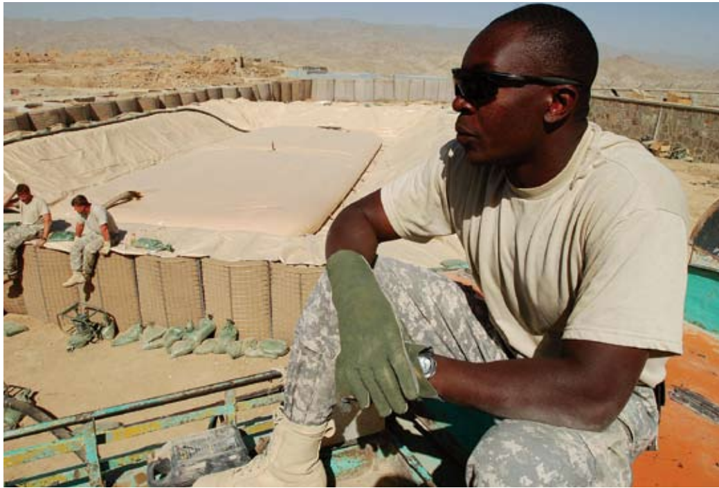
A Soldier sits on top of a fuel truck watching a newly constructed fuel farm being filled.
