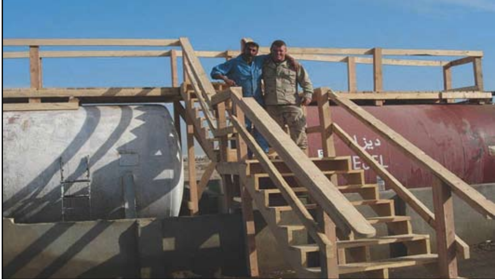
This fuel bridge, built by Soldiers of the 16th CSG, permits safe fuel transfer to skid-mounted tanks.
