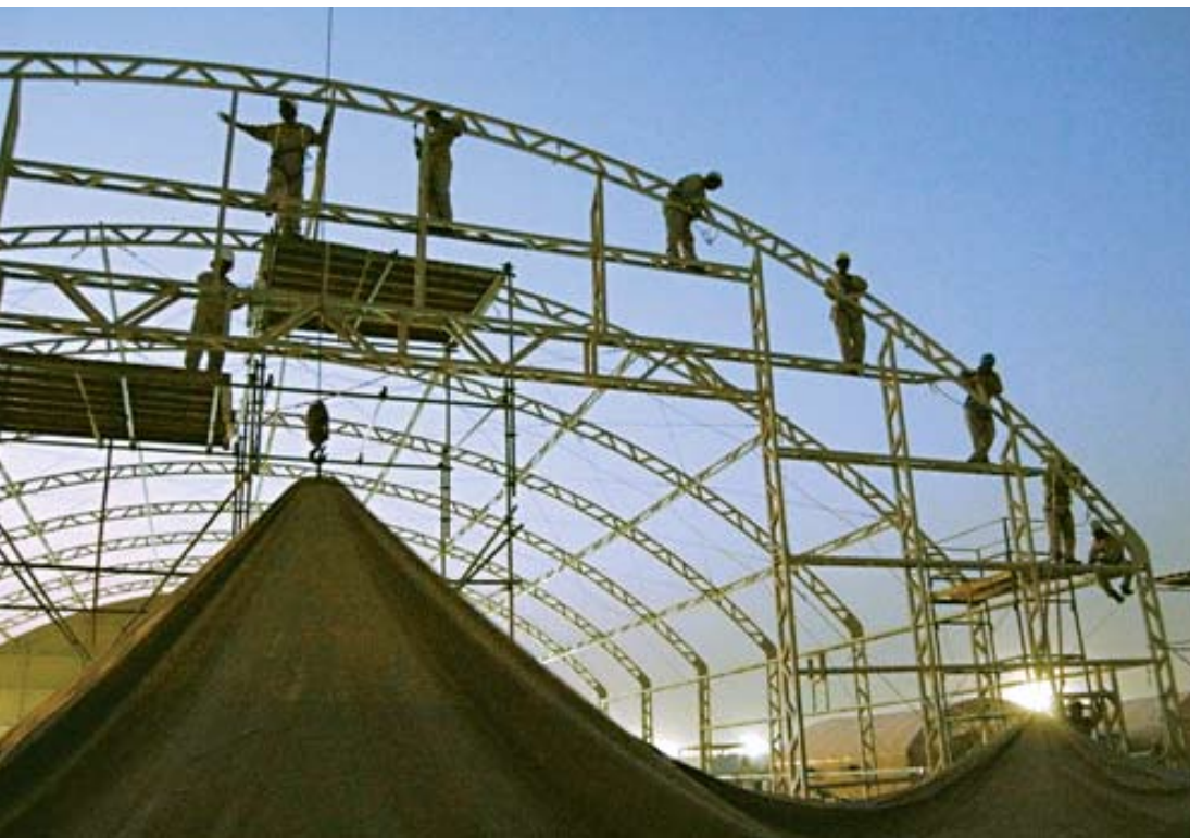
As darkness falls, Army contract employees install a fabric end section on a new maintenance tent at Camp Arifjan, Kuwait. The tents are one way to protect Soldiers, civilians, and equipment from the sun, wind, dust, and high temperatures of the Arabian Peninsula. (Photo by Jim Hinnant, 401st Army Field Support Brigade)
