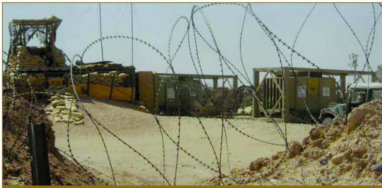
Concertina wire sits atop the berm that surrounds a pump station. To the left, 20-foot MILVANS used as an operations center are sandbagged to provide protection from small arms and indirect fire fragmentation. The 800-gallon-per-minute IDPS pumps are at right.
