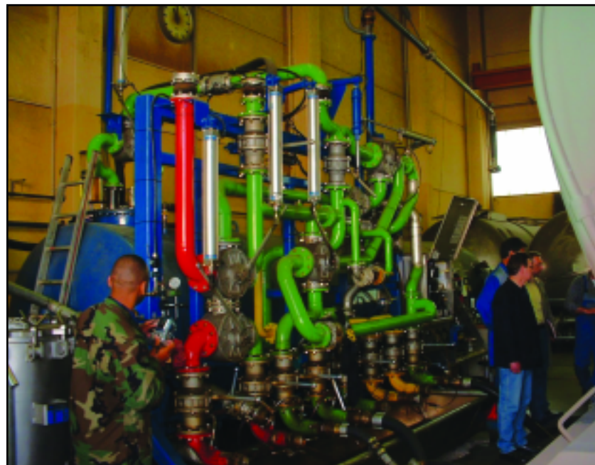
This hydrostatic test apparatus is used to test Army tankers at Industriewerke Saar GmbH.
