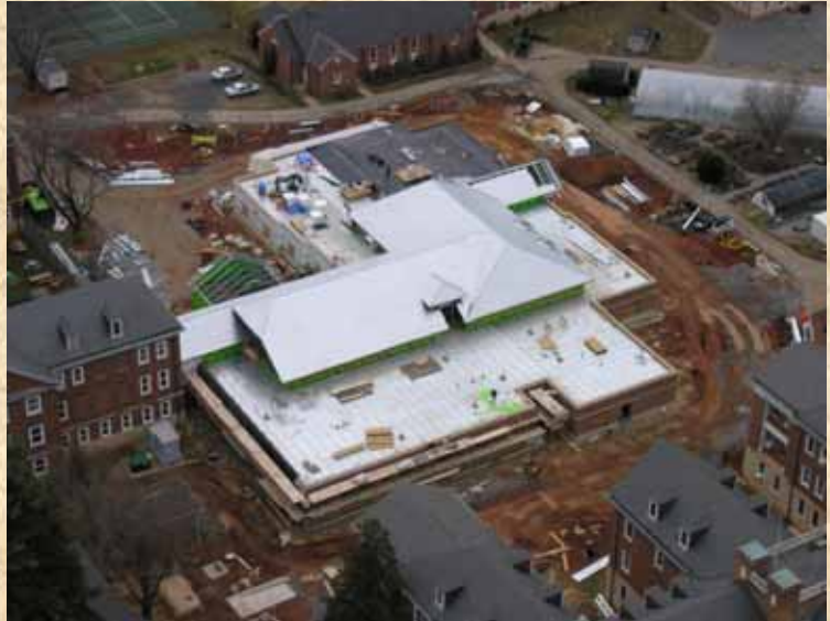
Aerial view of Building 8 Addition—Photo by Ricky May, SkyShots Helicopters. Used with permission by Hanke Constructors.
