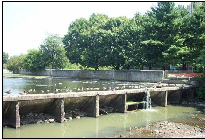
Dam 1: Main Street Dam, river mile 0.72. The 9.3-foot dam prevents fish passage.
