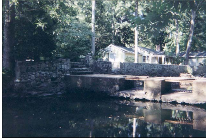
Dam 3: North of Arden Lane, river mile 5.22. Base of dam blocks fish passage.
