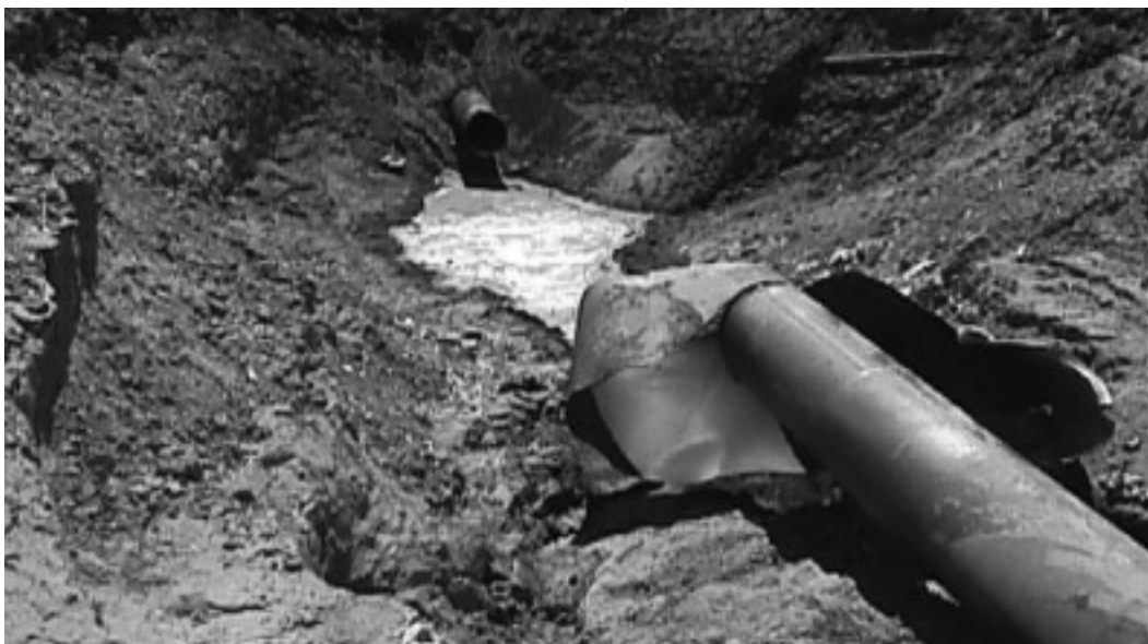
Crater created by pipe rupture.
