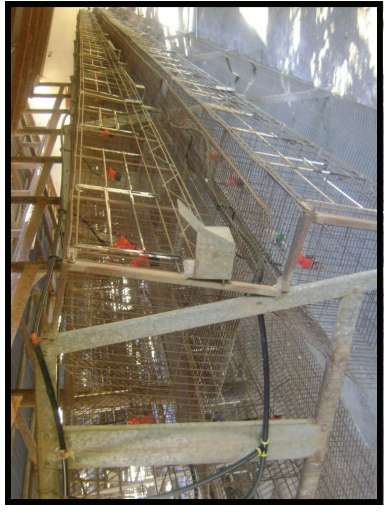
Shibani Multi-Purpose Cooperative - poultry shed (top), poultry shed under rehabilitation (bottom)
