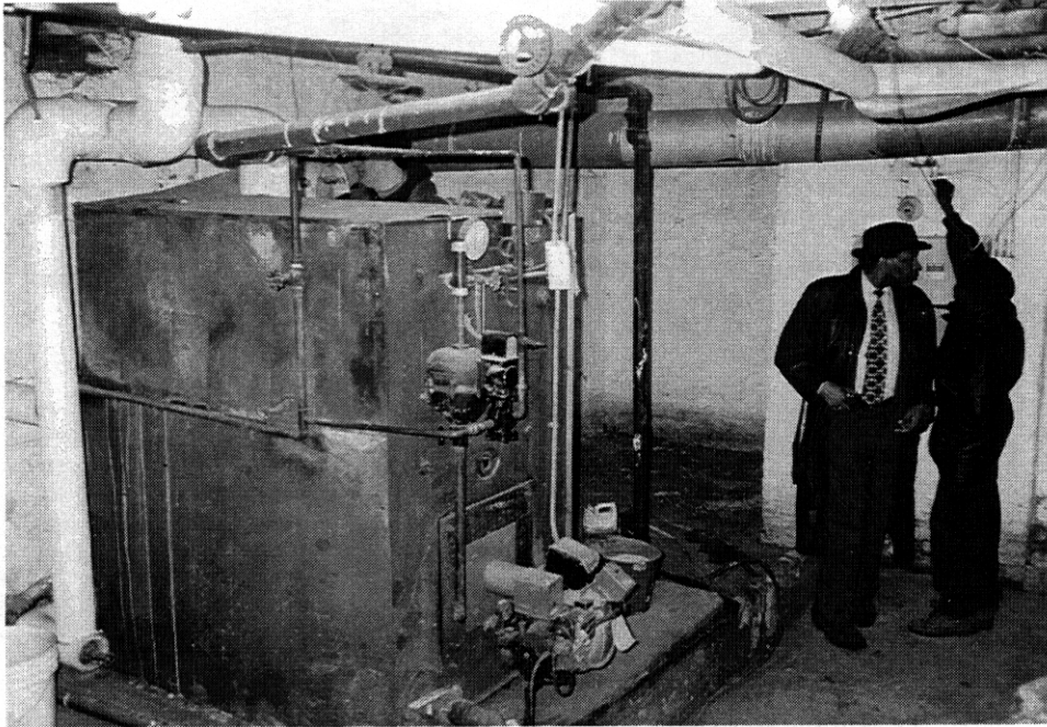
Fig. 2.16. Newly insulated distribution pipes at an existing heating system.
