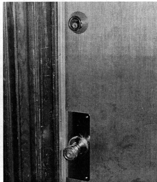
Fig. 37. New door-locking mechanisms and weather stripping provide security and lower convective losses.
