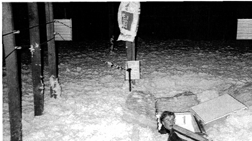
Fig. 6.6. A completed attic insulation job in an apartment building. Blown cellulose is used except in the hatchway area, where fiberglass batts provide a better, cleaner fit. The empty bag near the hatch provides product information for inspectors and others.
