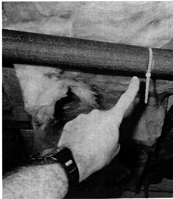
Fig. 36. When basement floors are insulated, it is all the more important to insulate pipes, both hot and cold.
