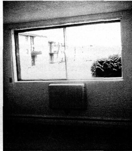
Fig. 5.5. Air conditioner covers are one of the few building shell retrofits regularly applied in the RAP multifamily program.
