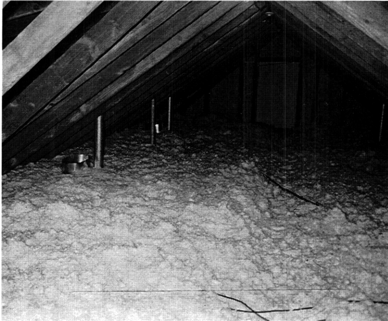
Fig. 6.15. Part of the finished attic insulation. The air from ventilation fans no longer comes into the attic.
