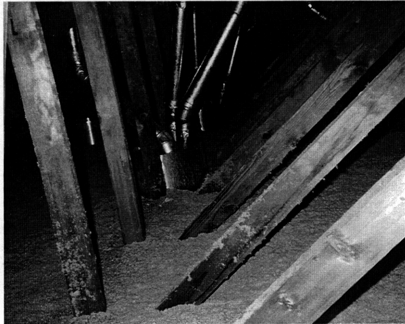
Fig. 6.21. It is difficult to prepare an attic for insulation when ventilation pipes are so closely interwoven with trusses.
