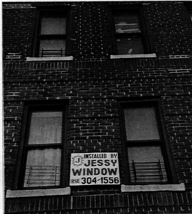
Fig. 2.31. New replacement windows were required to make this building habitable.
