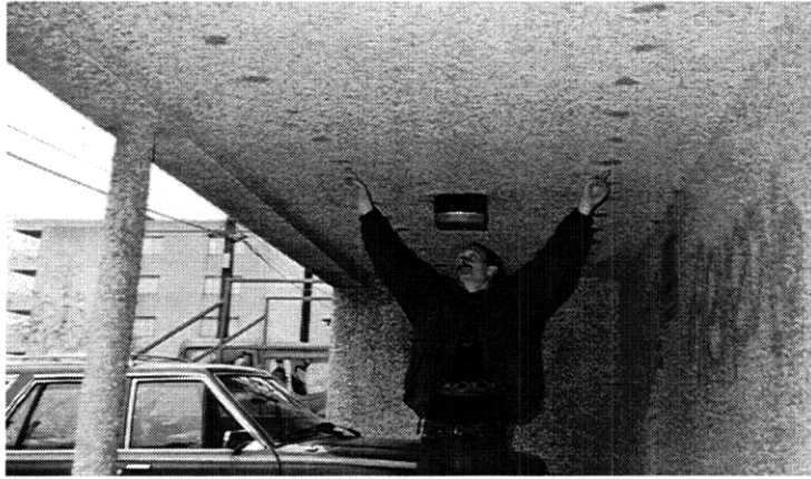
Fig. 6.22. Vince Feltes points out where holes were made to accommodate the hose for blowing cellulose in the overhang area.
