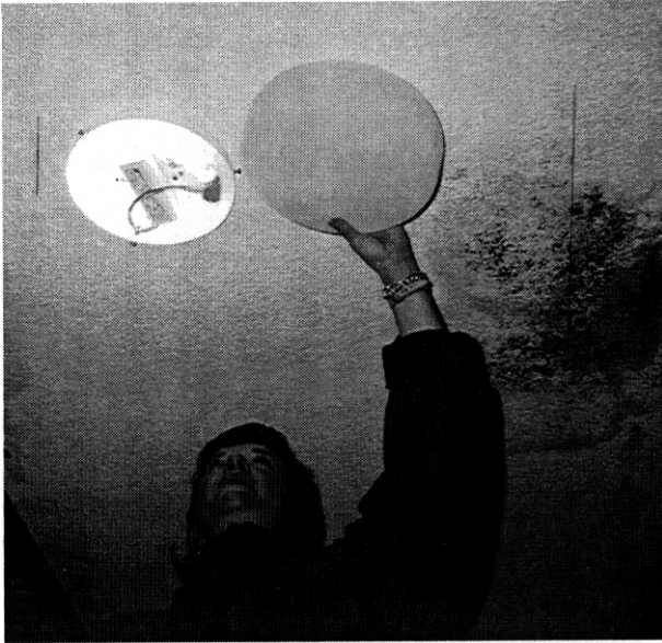
Fig. 6.17. Gail Travers, of the Department of Housing and Human Services, examines fluorescent fixtures installed at the Lam-Bow apartments. Note the evidence of a moisture problem (now cured) in the ceiling.
