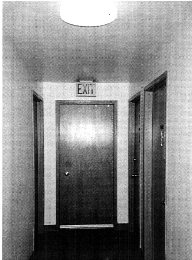
Fig. 6.23. The exit doors at the end of the common hallway were weatherstripped and new energy-efficient light fixtures installed.
