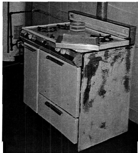
Fig. 3.14. Heat for the apartment is provided by this combination unit. Hot water units are located within each apartment.
