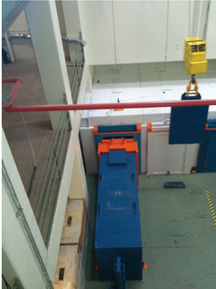
Figure 3–50: Photo of cask-to-morgue cell transfer system used at C-0 Remote Handling Facility
