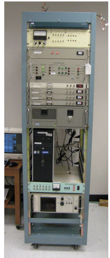
Replicated Master Station hardware in the EMF lab.
