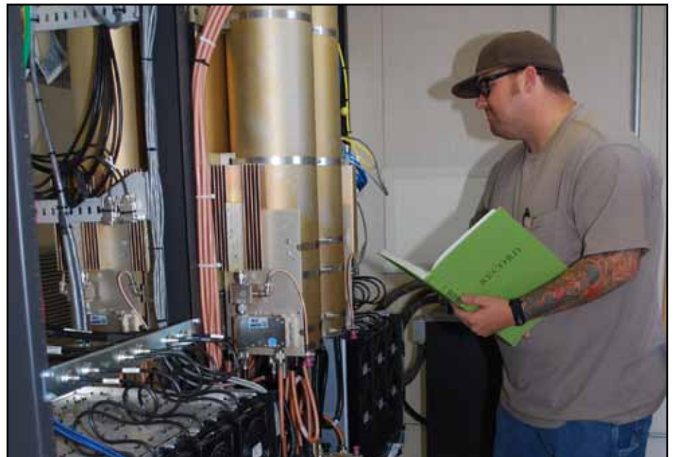
Bret Moore, NEC electronics technician, explains how the new system is much more compact, faster and reliable. (Photo by Mary Flores)
