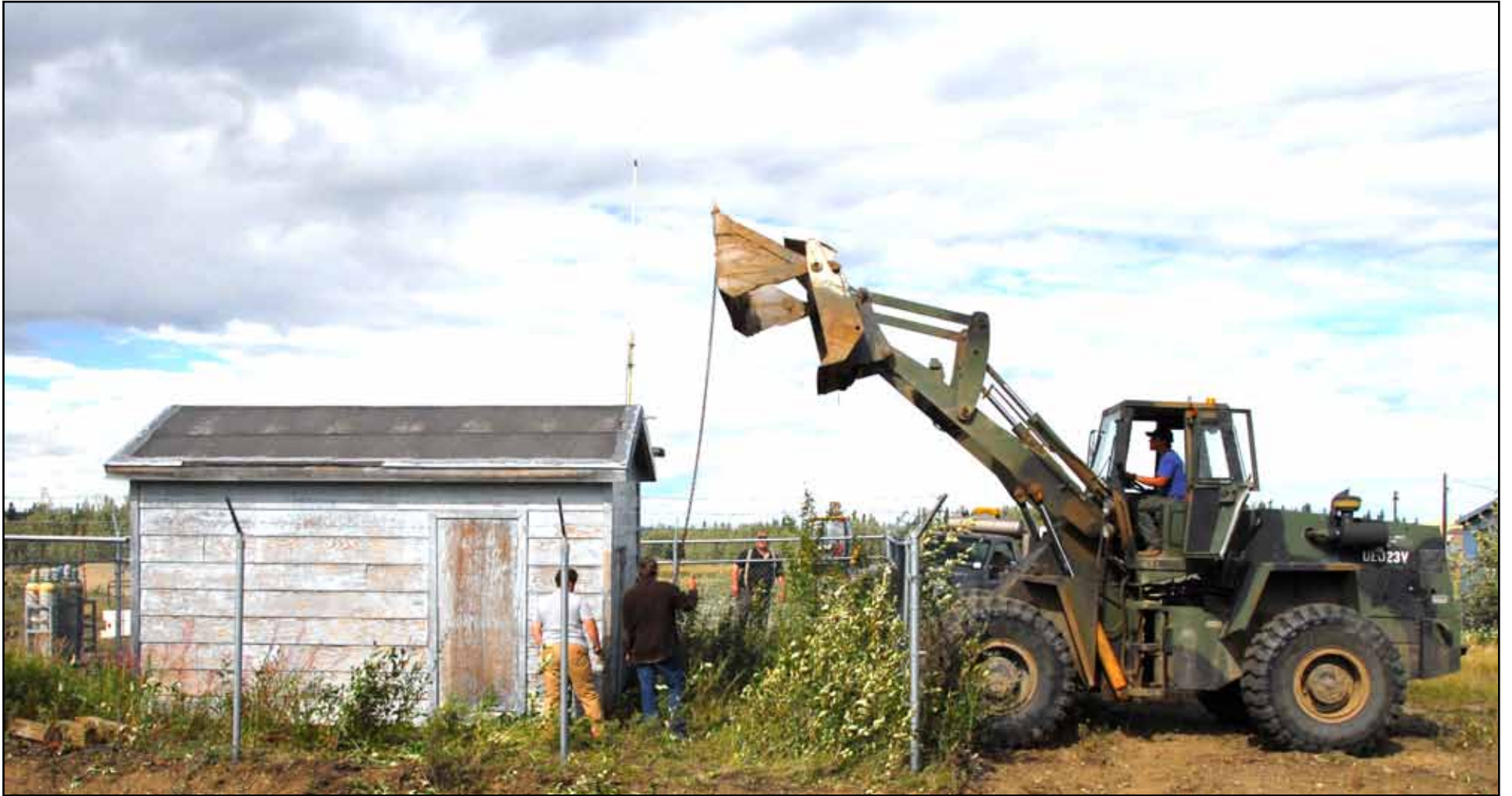
From left to right, CRTC employees Dan Wozniczka, Garry Garner, Wayne Robertson and Russell Hollembaek use heavy machinery to lift a meteorology building onto steel support beams. Alaska's freezes and subsequent thaws often cause structures like this to sink into the ground. "Because of our remoteness and many competing demands, it is not always possible to get the necessary, timely support from the department of public works to work on these types of projects," explained CRTC commander Lt. Col. John Cavado. "Approved self-help orders and CRTC's rugged professionals going above and beyond their regular duties enable us to remain mission ready." (Photo by Mark Schauer)
