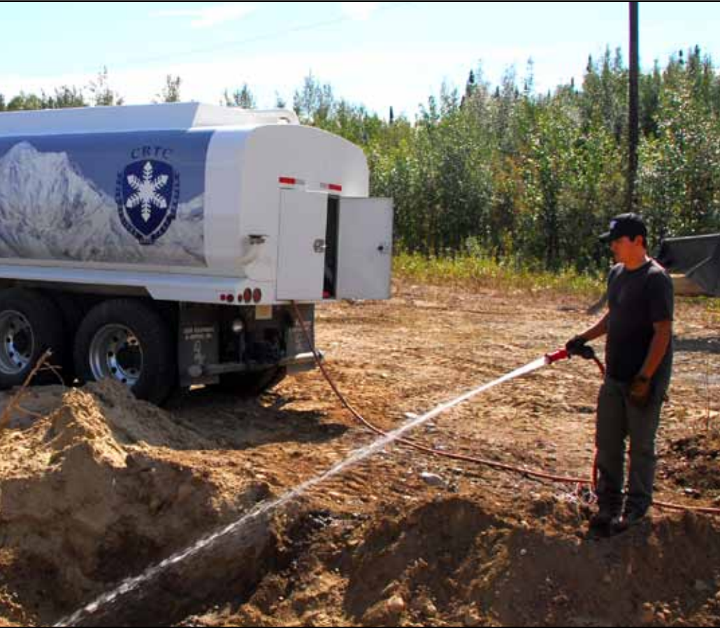
...an electrical conduit leading to one of the CRTC meteorology team's three new stations. Any type of construction is difficult or impossible to complete in winter, when the ground is frozen.
