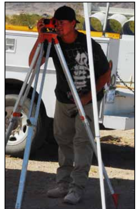
Maintenance crews are trained in a variety of skills including using surveying tools like this one.
