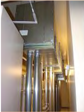
Heat Recovery from Dryer Vents
