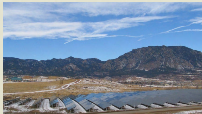
Fort Carson photo-voltaic
