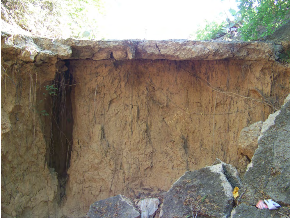
Figure 11. Soil profile exposed under collapsed roadway west of Growdon Road, looking east.
