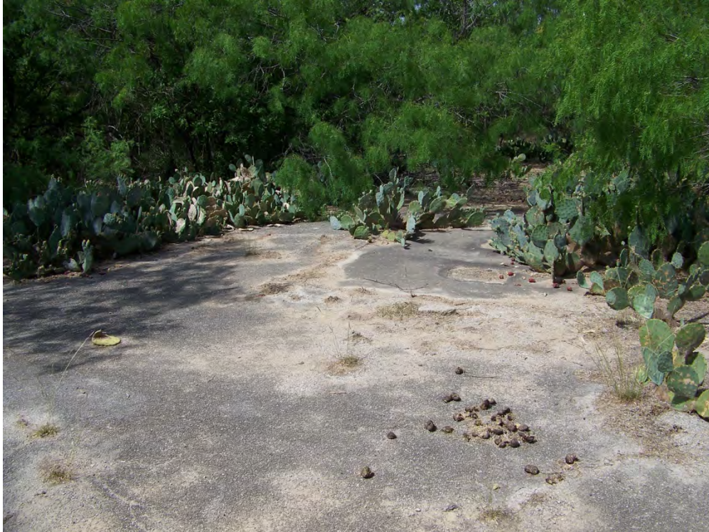
Figure 12. Remnants of an asphalt parking lot/road west of Growdon Road, looking west.
