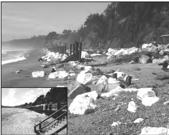
Figure 1: February 1983 photograph of the remains of a wooden seawall at Seacliff State Beach. Waves generated by the 1982-83 El Niño destroyed the seawall and scattered the large stones that had been emplaced seaward of the wall. Insert: April 1985 photograph of the replacement seawall and rebuilt beach. That seawall remained intact through the 1997-98 El Niño.
