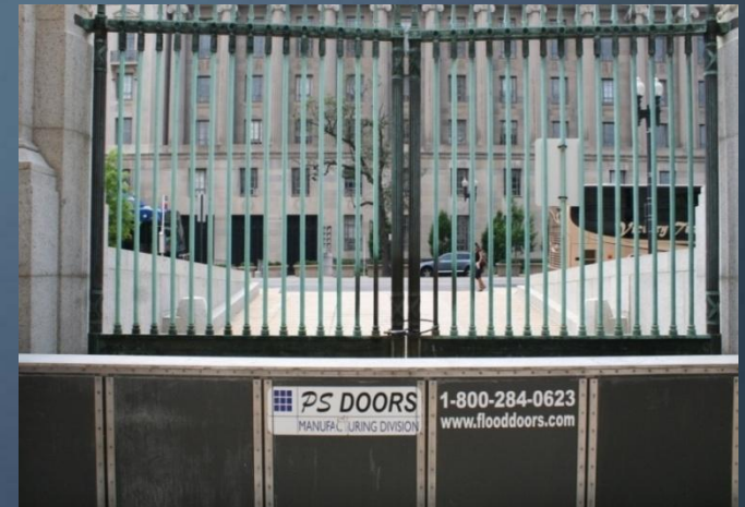
Self-rising flood gates at the National Archives, an example of a site-by-site solution
