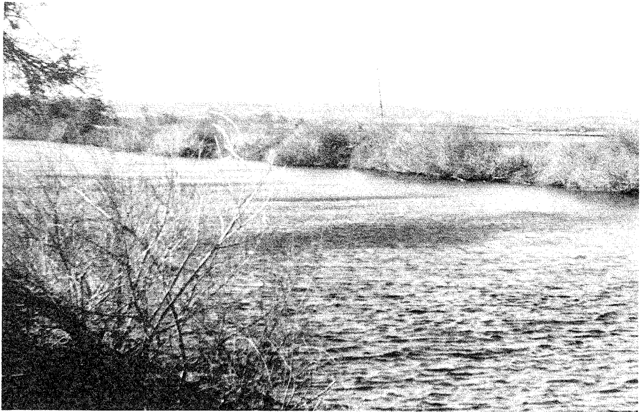
Figure 5. Privately owned and maintained levees on Sevenmile Slough. Note steepness of edge, erosion, and narrow riparian band extending into water.
