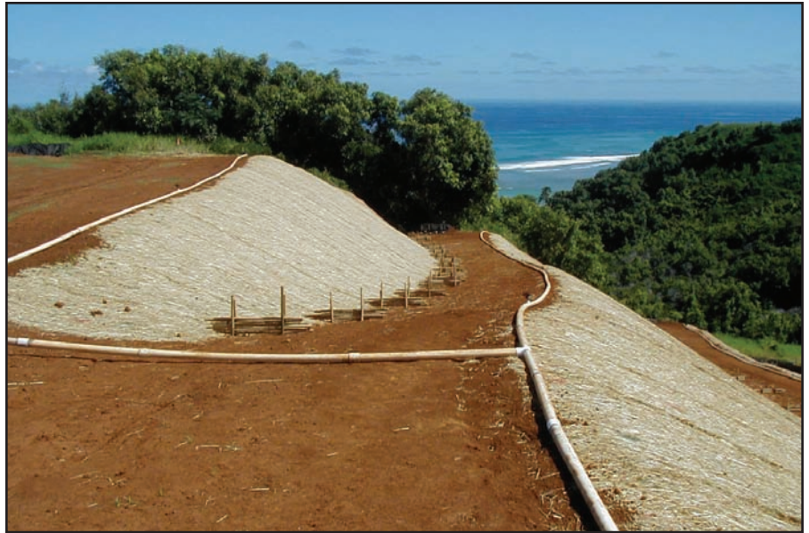
Figure 9.8. This steep roadcut at a construction site on Kauai is vulnerable to erosion and movement of sediments to the beach and nearby coral reef ecosystems. Practices to stabilize the slope include terracing, erosion control matting, hydromulch, and wattles. Photo: W. Wiltse.
