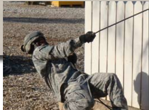
Spc. Lacy Thompson, B Company, 44th ESB, pulls fiber cable off a reel in support of the Fiber Installation Mission on Forward Operating Base Delta, Iraq.
