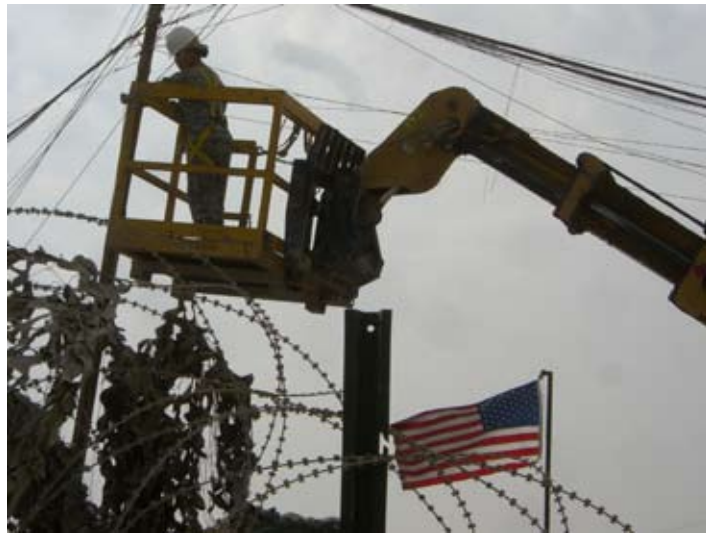
Cpl. Veronica Cruz, C Company, 44th, repairs communication cable at Forward Operating Base Echo in Iraq.
