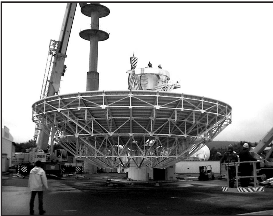
Workers installing the AN/FSC-78B Antenna at the DSCS site in Landstuhl, Germany.
