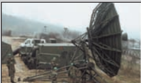
The 86A team finalizes antenna installation and prepares to access the satellite during Agile Lion 2001.
