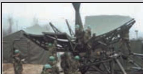
The Landstuhl TSC-86A team, 43rd Signal Battalion, from the DSCS Station bolts on a SATCOM panel during the installation of the AS-3199 antenna in support of SETAF during Agile Lion 2001.
