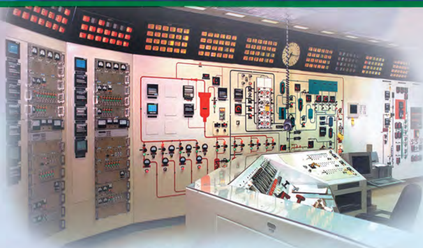
HFIR Control Room
