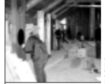
Top left: Several volunteers raise a wall plank into place. Above right: A retired builder and soil scientist, an engineer, a dairy farmer, and a rancher join forces to work on an ADA-accessible entrance to the building.
