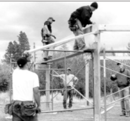
Inland Northwest Associated General Contractors of America erect an environmental education shelter.
