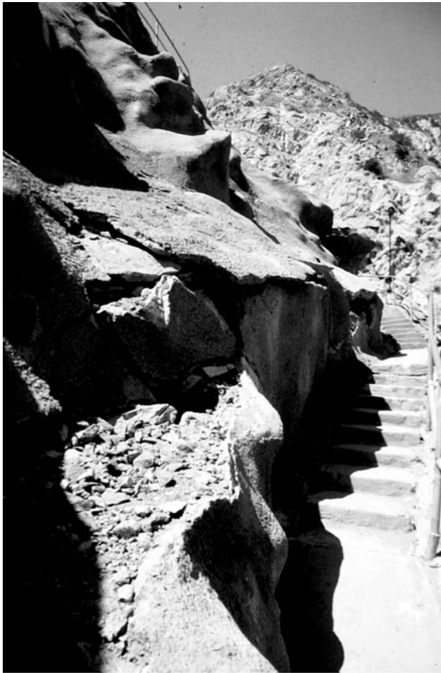
Figure 5. Close-up of fractured rock slopes and shotcrete facing near Pacoima Dam.
