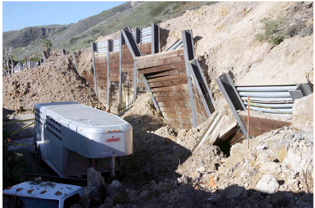
Fig. 10 Steel-and-timber wall built after the 1995 landslide was overtopped and tilted forward in places by the 2005 landslide
