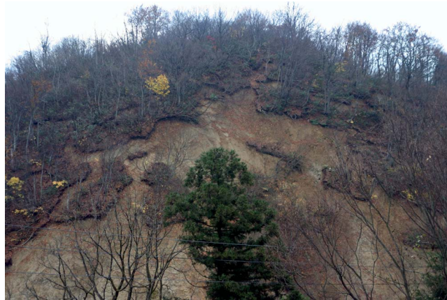
Figure 10. Slope whose soil mantle was stripped off by strong shaking.
