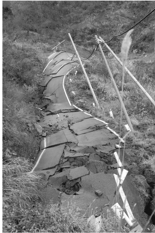
Figure 29. Landslide damage to a roadway east of Yamakoshi. Note the backward rotation of the roadway and utility poles in the foreground, together with their forward rotation in the background.
