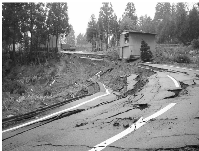
Figure 7. Looking northwest on Highway 291, toward the same fire truck as in Figure 5. In the foreground is an additional roadway section destroyed by landsliding.
