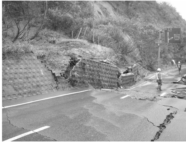
Figure 28. Landslide damage to a retaining wall and adjacent roadway on Highway 291, south-east of Yamakoshi City Hall.
