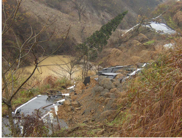
Figure 21. Damming of a tributary valley caused by rotational slides and roadway embankment failures in the Yamakoshi epicentral area.
