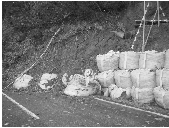
Figure 4. Slide debris deposited on sandbags that had been placed to stabilize a pre-existing rainfall-induced landslide along Highway 9 east of Nagaoka.
