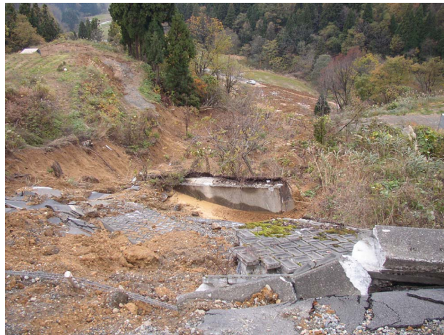
Figure 5. Damage to the roadway and to a retaining wall on Highway 9, east of Nagaoka.
