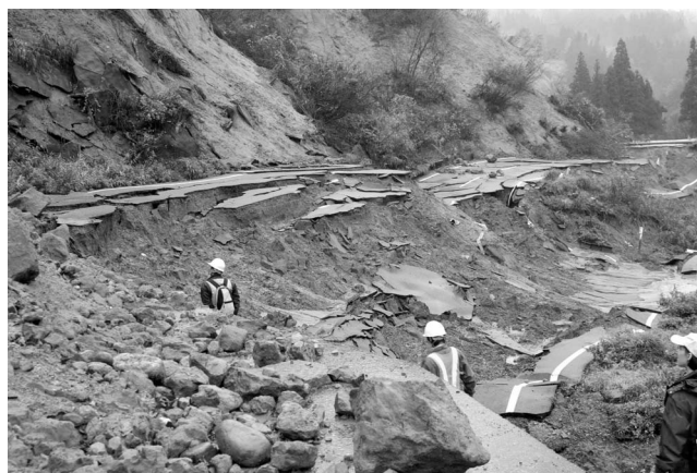
Figure 27. Failure of a roadway embankment fill south of Yamakoshi.
