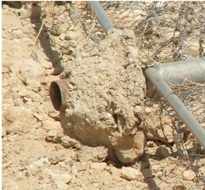
Site Photo 6. Concrete anchorage at failed fence post
