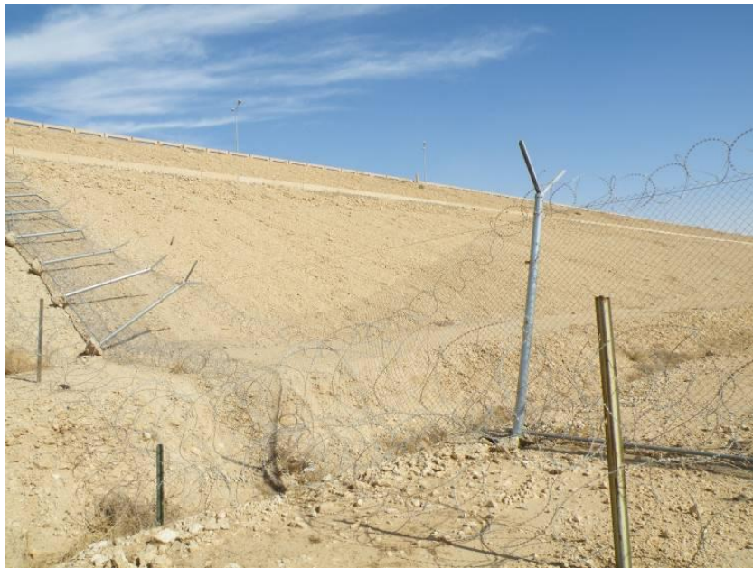
Site Photo 8. Poorly constructed swale crossing
