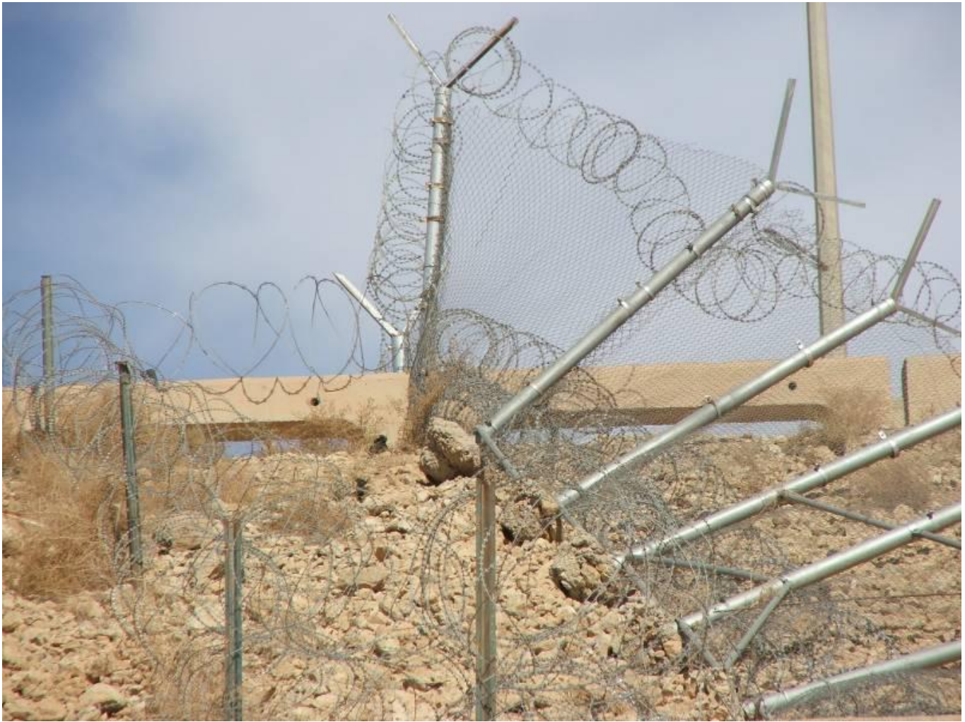
Site Photo 5. Failed fence section, upper end
