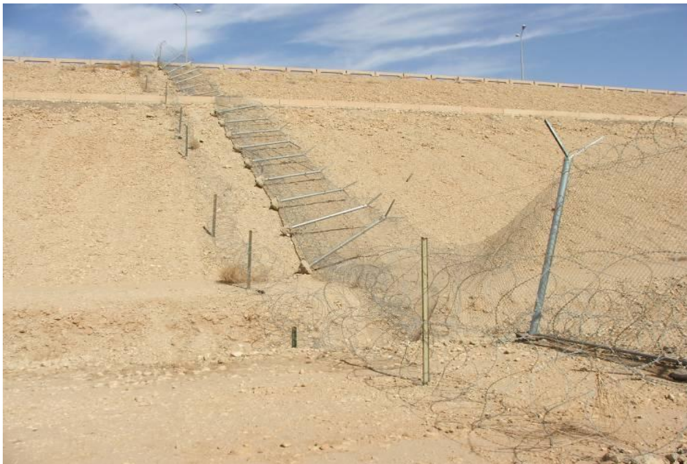
Site Photo 4. Failed fence section
