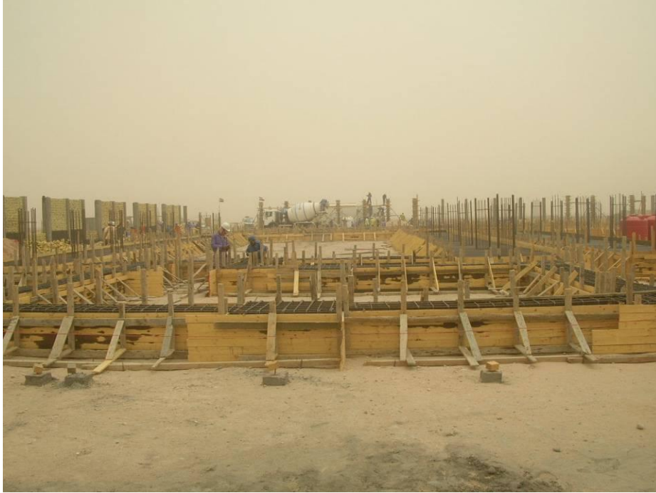
Site Photo 5. Strip footers tied together at the base (Courtesy of GRS)
