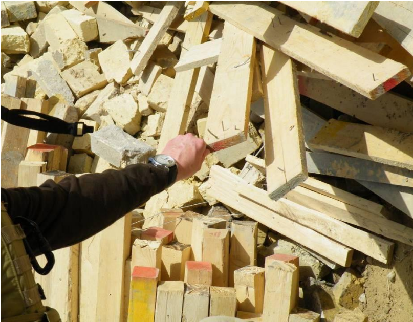
Site Photo 8. Project site littered with building materials
