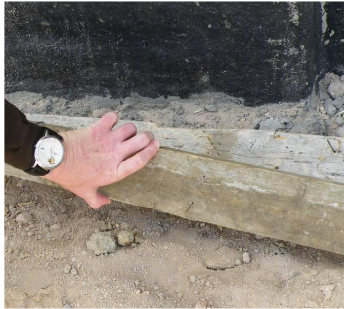
Site Photo 9. Protruding nails from formwork boards
