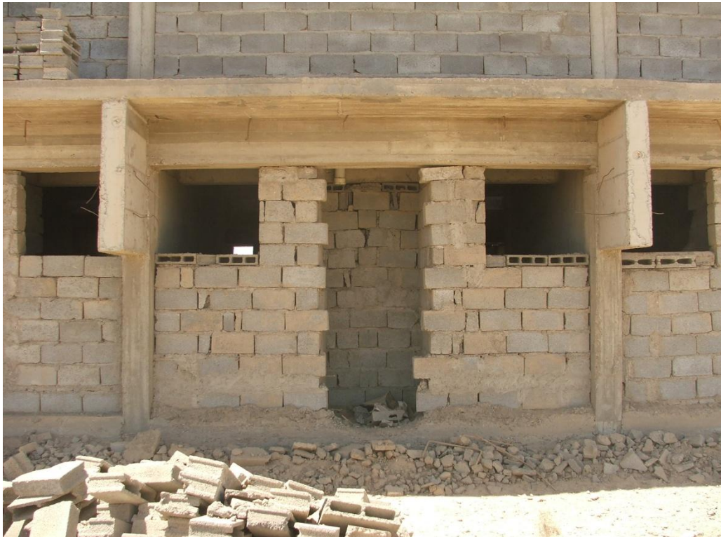
Site Photo 19. Example of poor block laying
