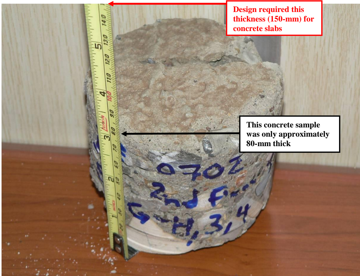
Site Photo 6. Measurement of a concrete core sample – design requirements specified at least 150-mm thickness; however, this sample was approximately 80-mm (Courtesy of the USACE)
