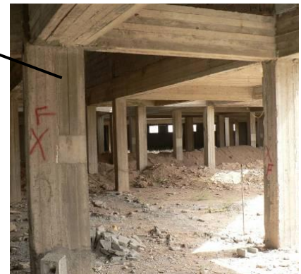
Site Photo 8. Location of low concrete strength (Courtesy of the USACE)
