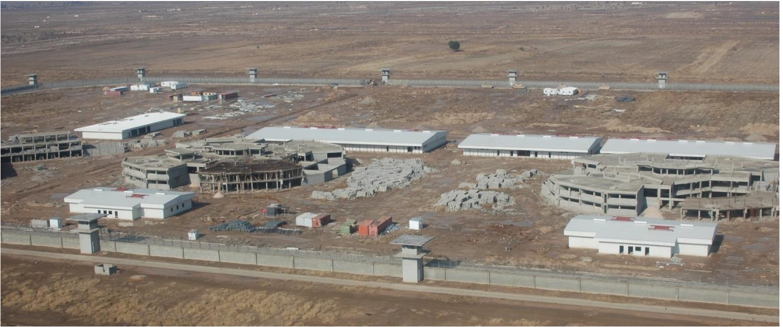
Site Photo 20. Aerial view of the KBS Correctional Facility from June 2007(Courtesy of the USACE)
