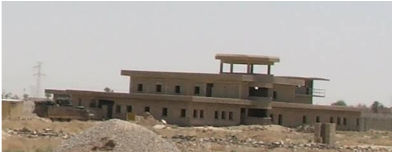
Site Photo 9. Still standing medium security building that the structural assessment recommended be demolished
