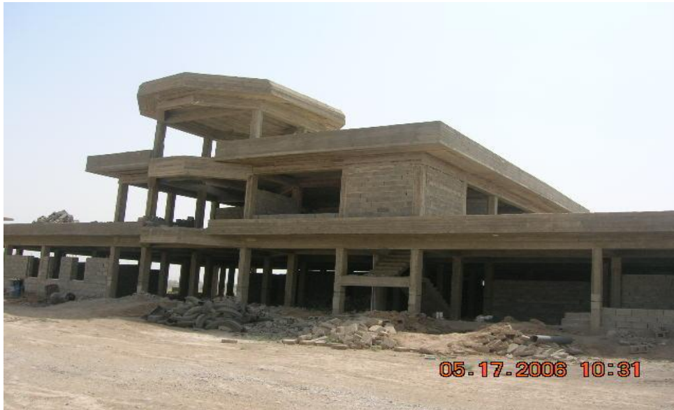
Site Photo 1. Status of construction at the time of Parsons' termination (Courtesy of the USACE)
