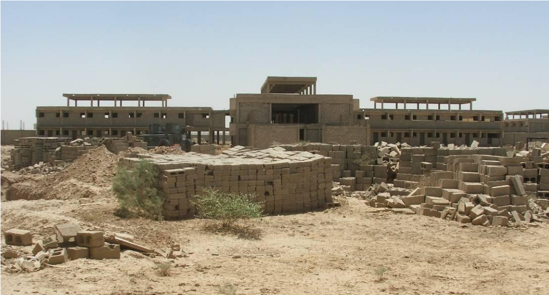
Site Photo 21. Concrete blocks still on site at the KBS Correctional Facility
