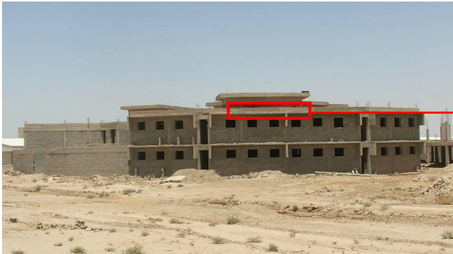
Site Photo 10. Medium security building that structural assessment recommended replacing
