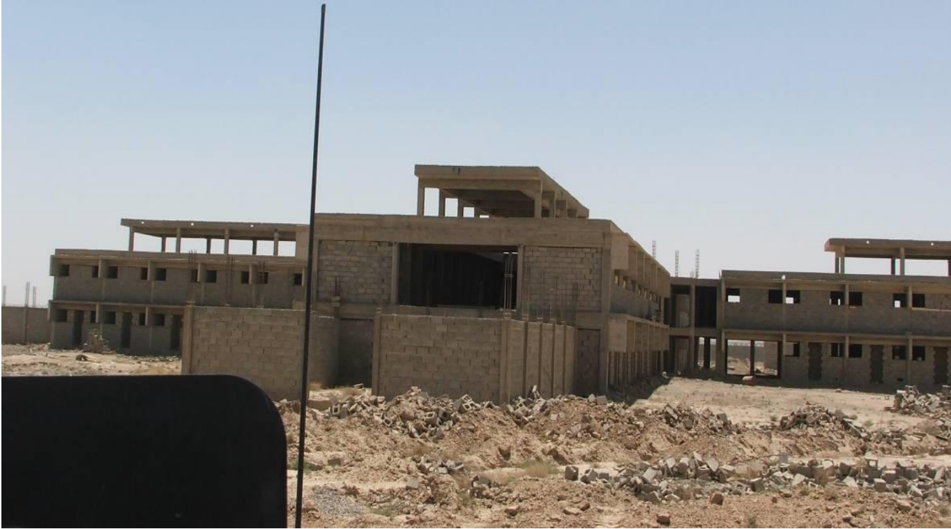
Site Photo 12. Exterior view of the maximum security building – no corrective action had been taken by the GoI
