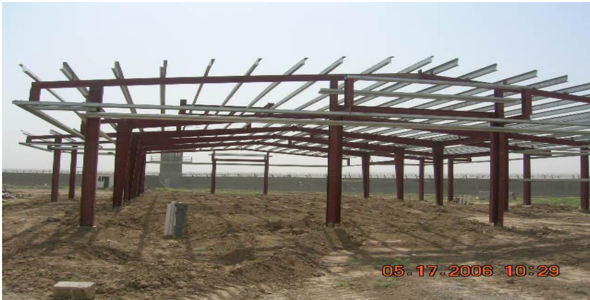
Site Photo 2. Status of construction at the time of Parsons' termination (Courtesy of the USACE)
