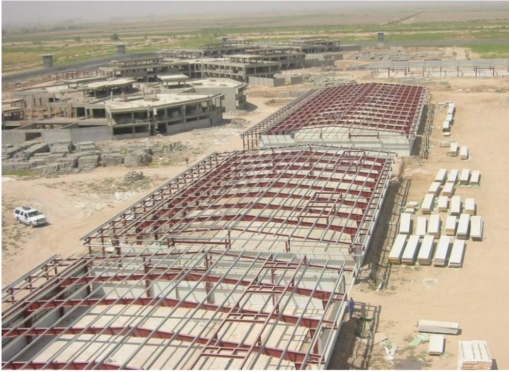
Site Photo 3. Status of project at the end of the bridge contract (Courtesy of the USACE)
