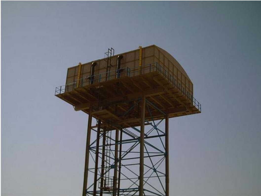
Site Photo 15. Elevated steel water tank after maintenance (Photo courtesy of USACE)
