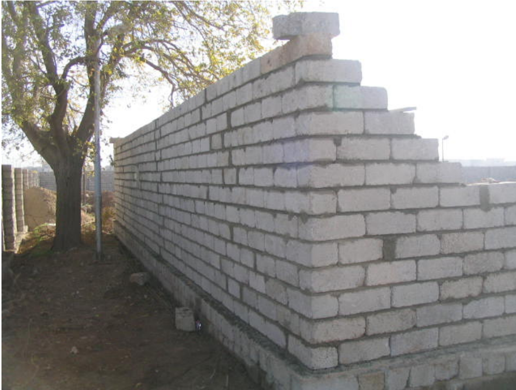
Site Photo 11. Construction of the manager of operations' new office (Photo courtesy of USACE)
