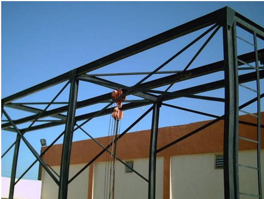
Site Photo 10. Installation of the new 3-ton crane (Photo courtesy of USACE)
