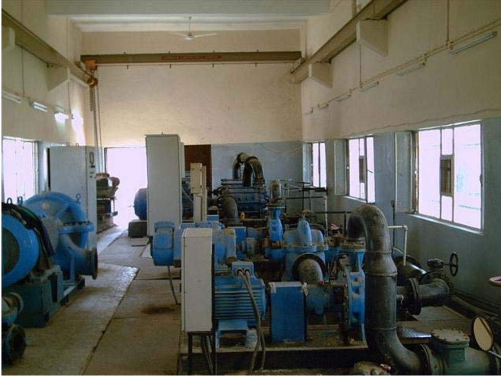
Site Photo 3. General maintenance performed inside the Bartilla Booster Pump Station pump room (Photo courtesy of USACE)
