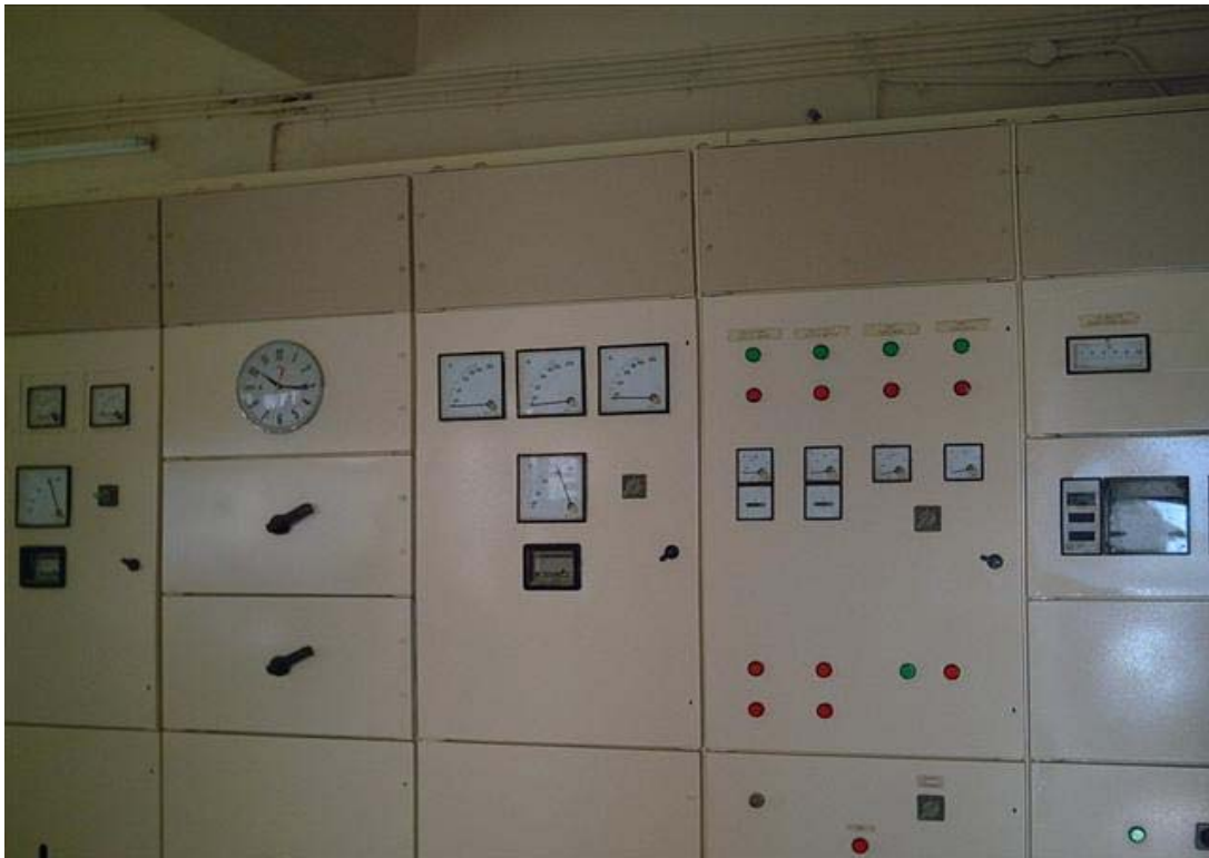
Site Photo 14. Pump house control panel after maintenance (Photo courtesy of USACE)
