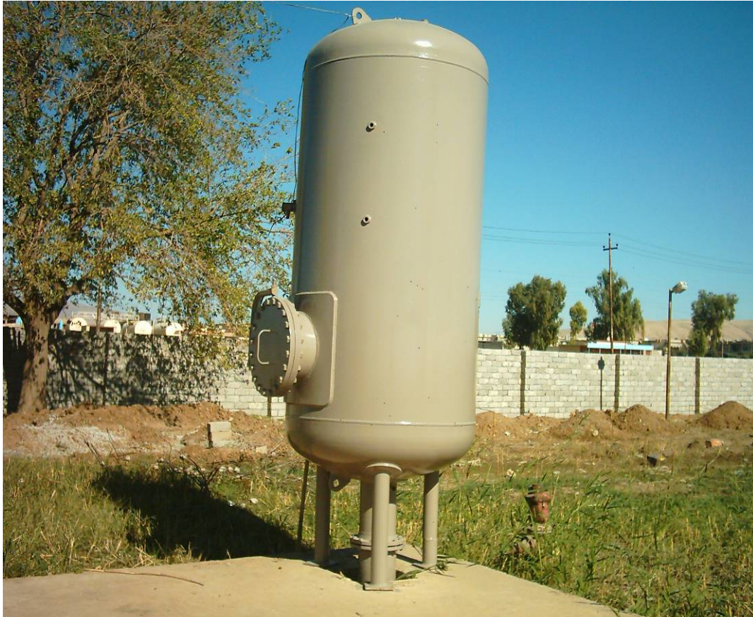
Site Photo 2. Anti-Hammer system after maintenance (Photo courtesy of USACE)
