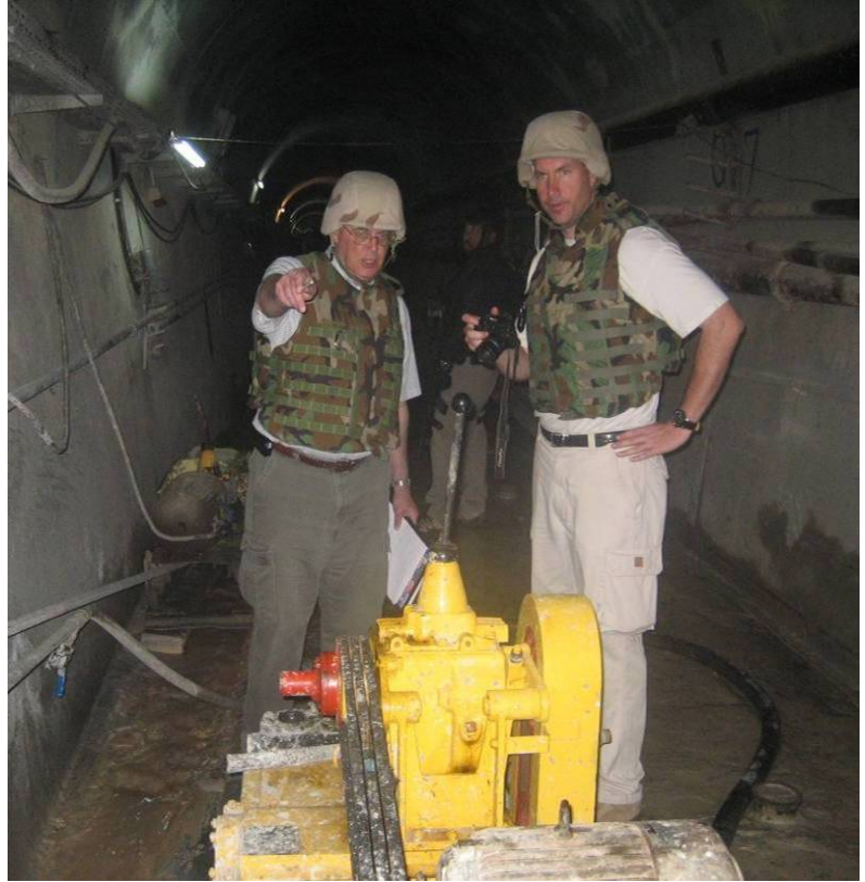
Site Photo 43. SIGIR inspector pointing out an active grout pump placing grout into a hole
