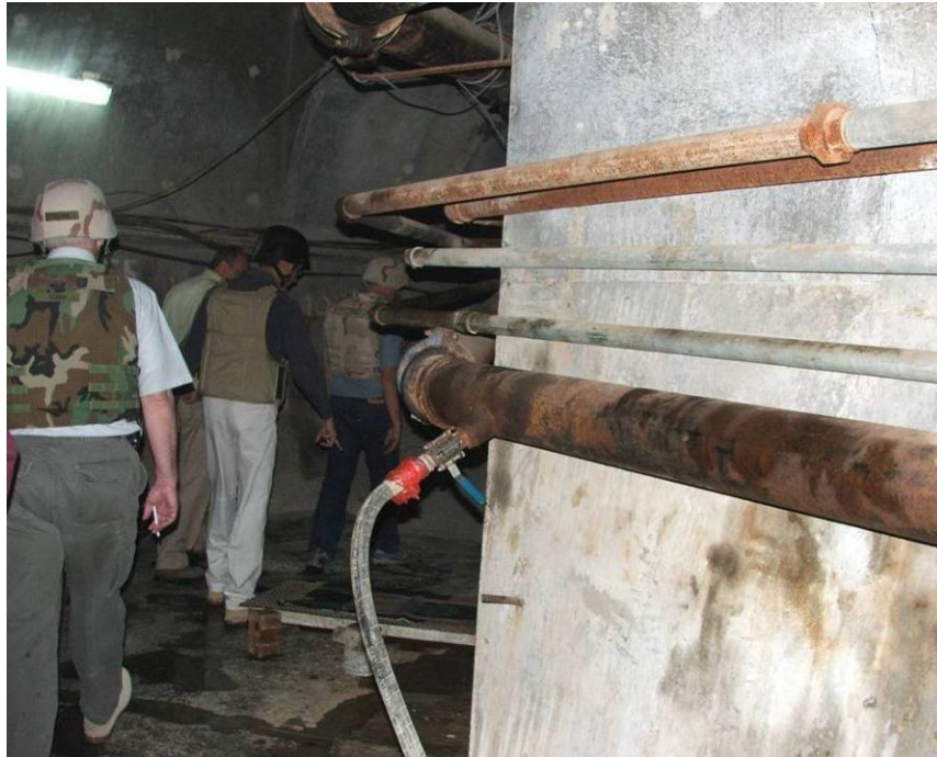
Site Photo 37. Partial view of the sharp right turn within the gallery tunnel
