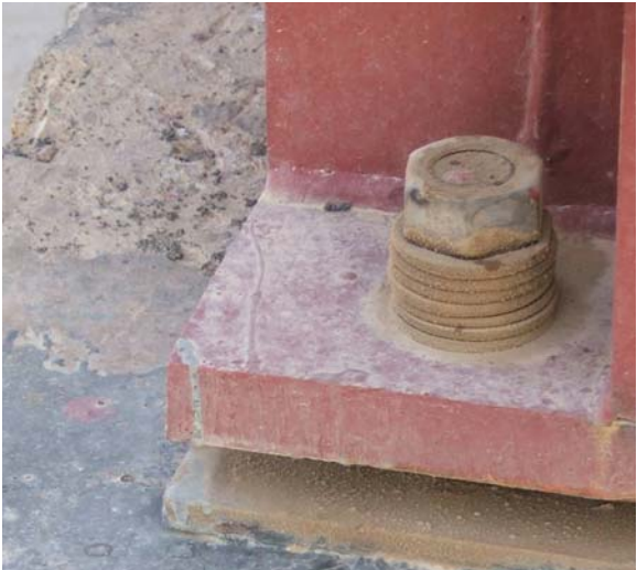
Site Photo 21. Poor installation technique (the use of 7 washers)
