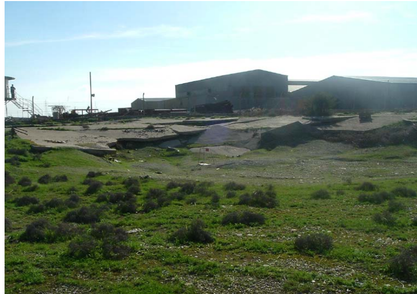
Site Photo 9. Sinkhole beneath a concrete-paved area (Photo courtesy of the USACE)
