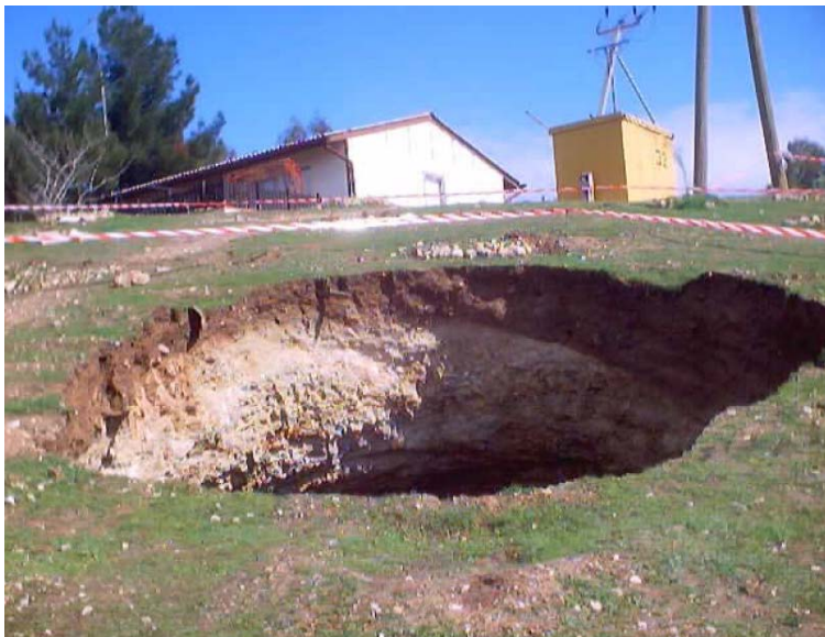
Site Photo 8. Example of a sinkhole (Photo courtesy of the USACE)
