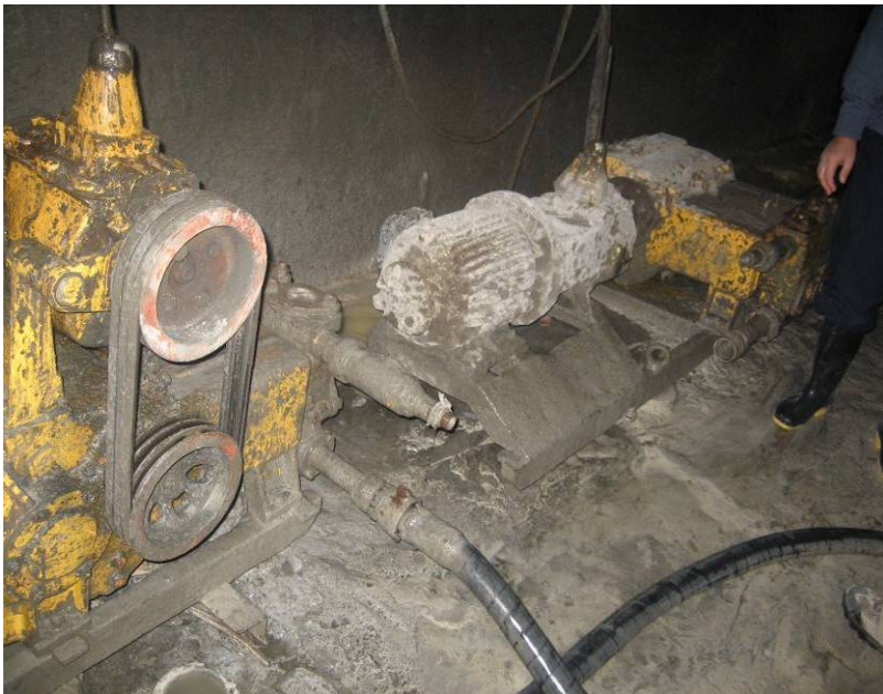
Site Photo 44. A grout pump actively placing grout into a hole (Photo courtesy of ITAO)
