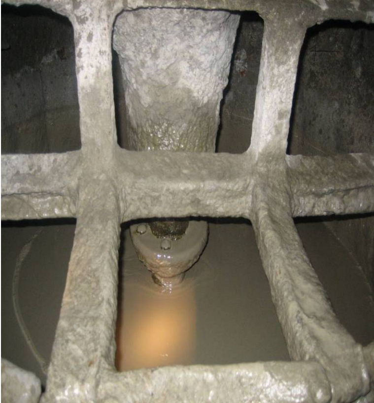
Site Photo 42. Existing agitator within the gallery actively mixing grout
