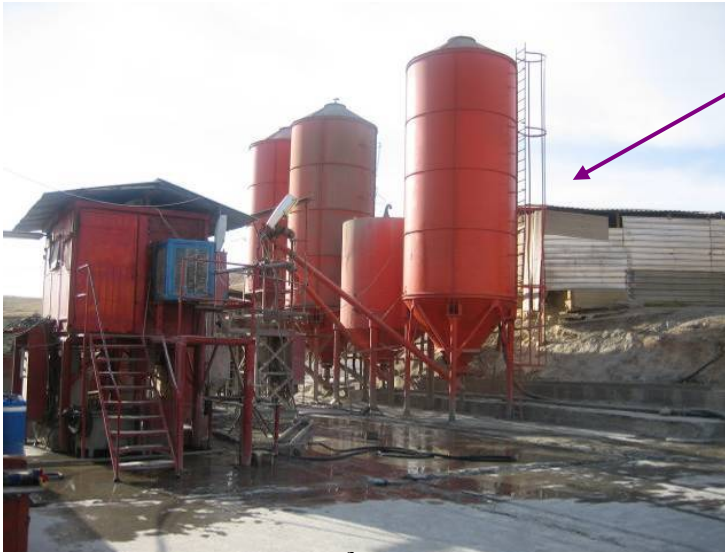
Site Photo 10. Existing 20- \text{m}^3/\text{hour} grout-mixing plant (Photo courtesy of the Iraq Transition Assistance Office (ITAO))
