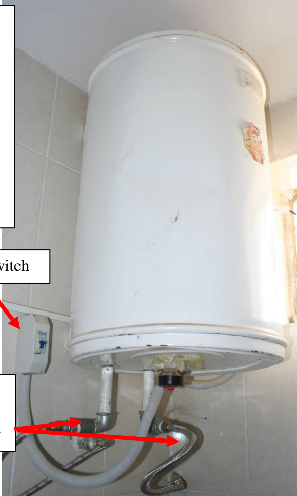
Site Photo 3. Water heater.
