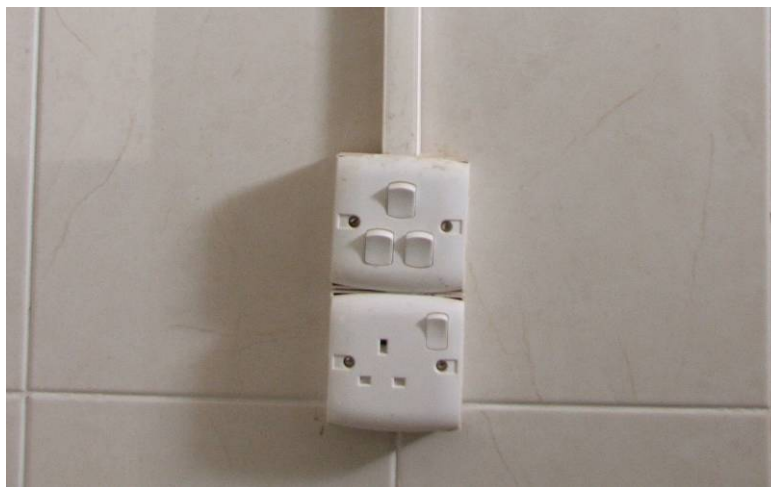
Site Photo 2. Throughout the facility wiring, switches, and plug-ins were securely fastened to walls as required by the SOW.
