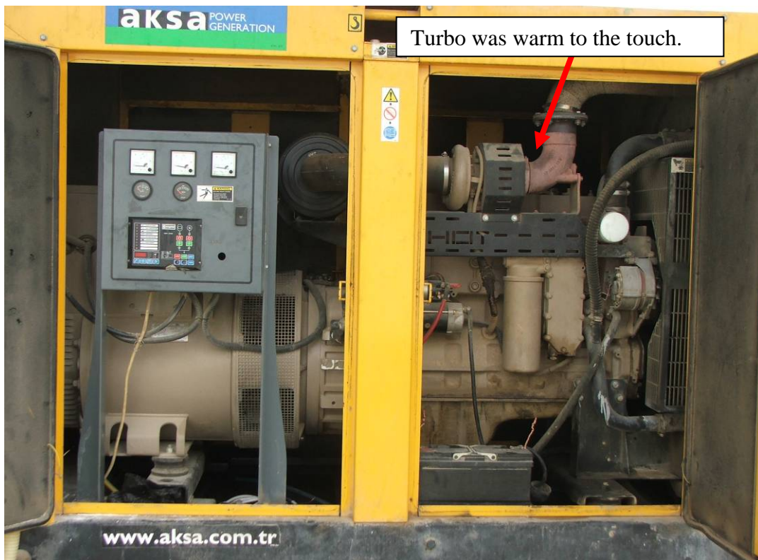
Site Photo 1. The generator installed per requirements appeared completely operational without any signs of neglect. When checked, the oil level was full and did not feel gritty. Belts and hoses appeared serviceable.
