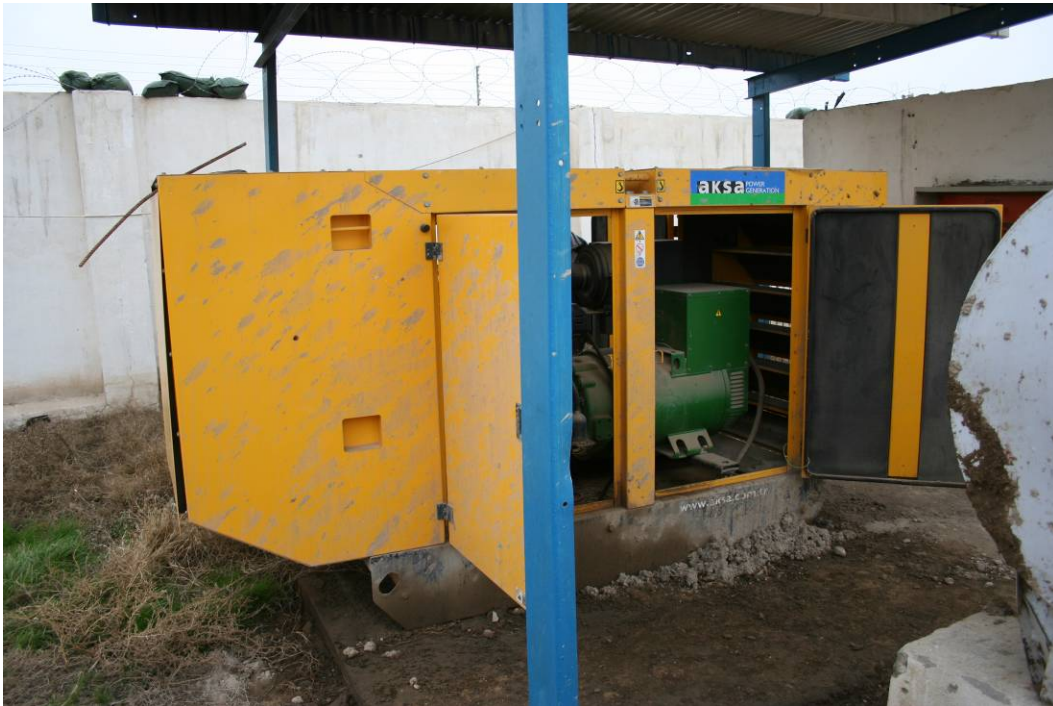
Site Photo 11. Without a fuel line and working controls, the new generator appeared abandoned.
