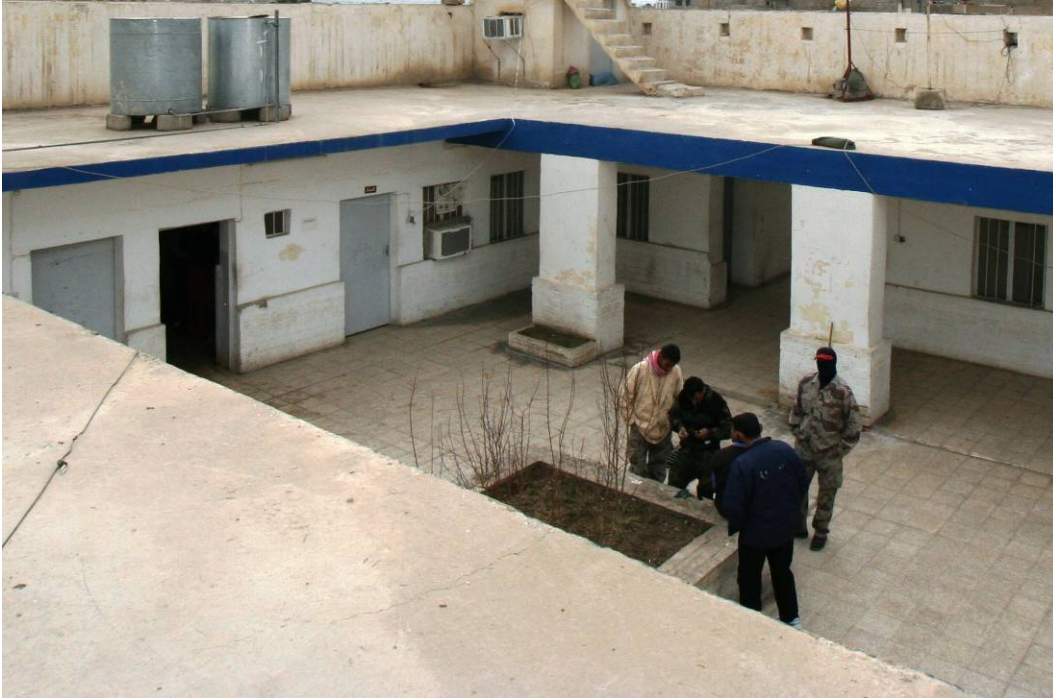
Site Photo 1. Observed condition of the same general area shown in USACE Construction Photo 13 appeared functional.
