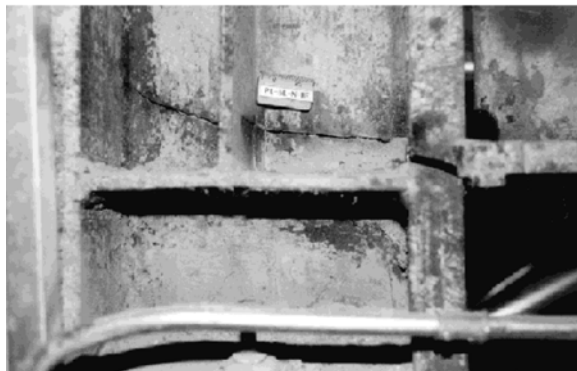
Figure 2-6 - Fracturing of W14 column at welded beam-to-column connection in Northridge earthquake.
