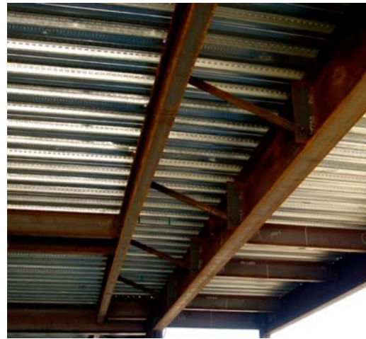
Figure 5-1 - Steel special moment frame beam stability bracing with a concrete filled metal floor deck.
