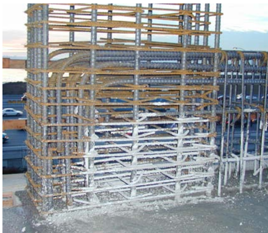
Figure 7-3 – Beam-column joint having multiple layers of beam reinforcement hooked at back side of joint. Note the upturned beam (the slab is cast at the bottom face of the moment frame beam).
