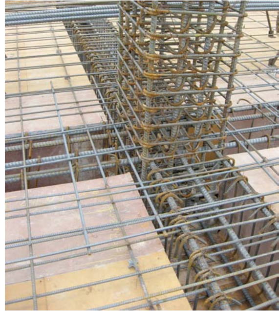
Figure 7-1 – Beam-column joint with beam corner bars swept to inside of column corner bars.
