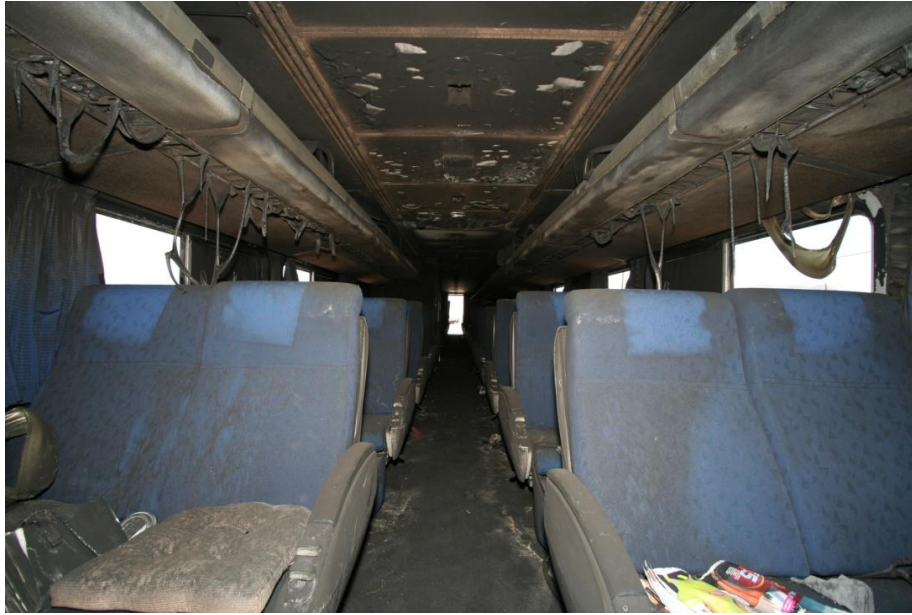
Figure 9. Photograph of interior of second coach railcar 35006, showing damage from heat and soot throughout.
