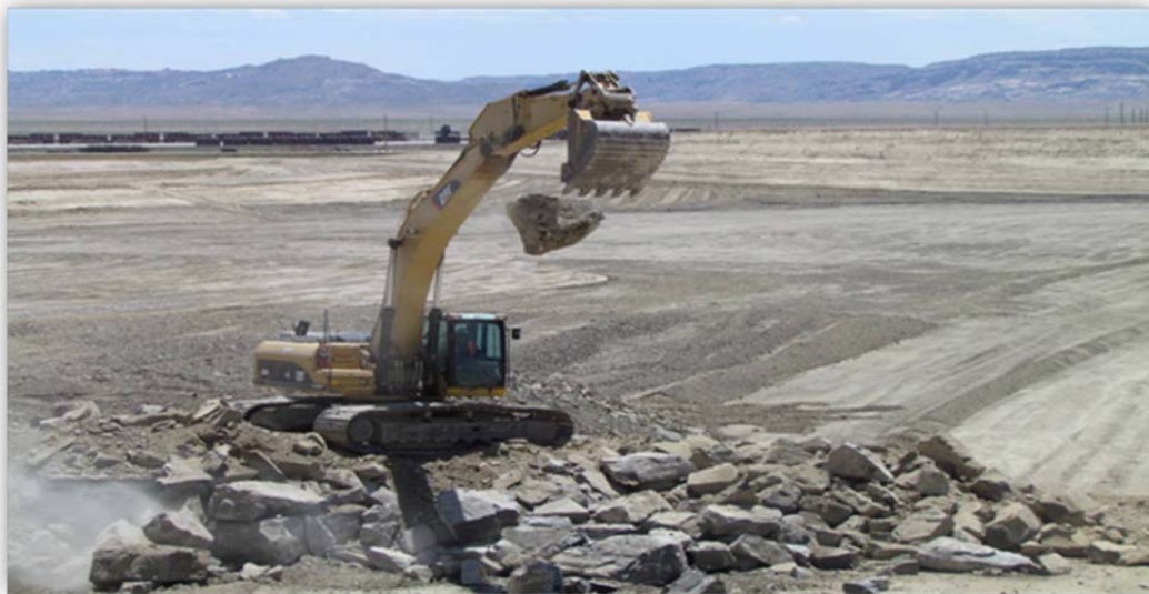
An excavator is used to break up limestone discovered during excavation of the second phase of the Moab disposal cell.
