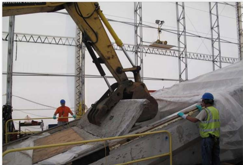
Removal of roof plug with excavator at the Brookhaven National Laboratory (BNL)
