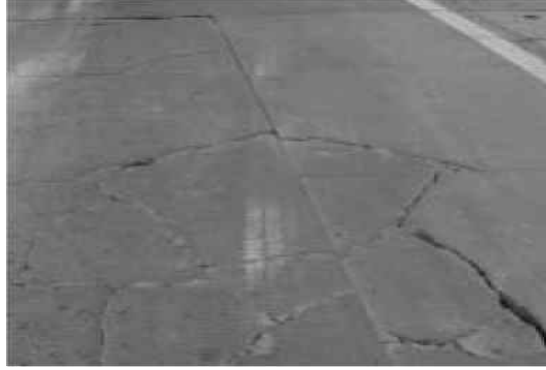
FIGURE 2-26. SHATTERED SLAB CONDITION
