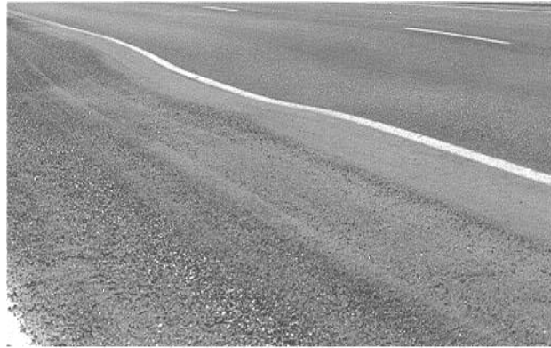
FIGURE 2-4. DEPRESSION IN PAVEMENT
