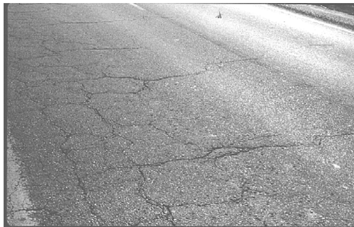
FIGURE 2-3. HIGH-SEVERITY BLOCK CRACKING
