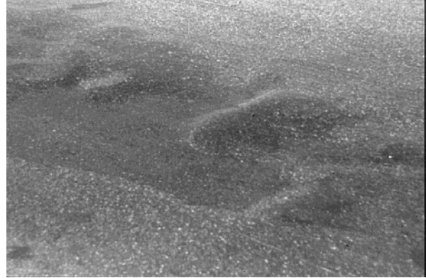
FIGURE 2-11. SHOVING IN A PAVEMENT
