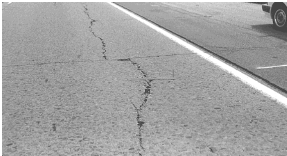
FIGURE 2-15. HIGH-SEVERITY LONGITUDINAL CRACKING
