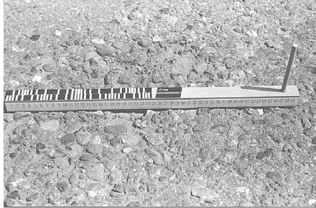
FIGURE 2-9. HIGH-SEVERITY RAVELING AND WEATHERING
