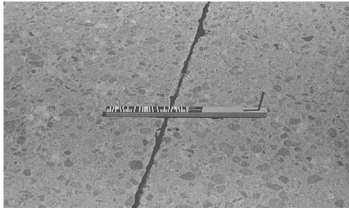
FIGURE 2-18. JOINT SEAL DAMAGE
