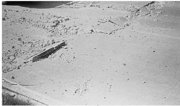
FIGURE 2-13. BLOWUP IN A PAVEMENT
