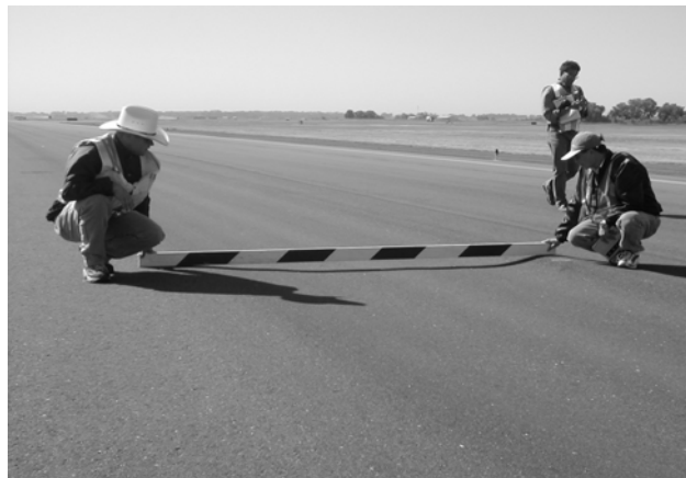
FIGURE 2-10. RUTTING IN A PAVEMENT
