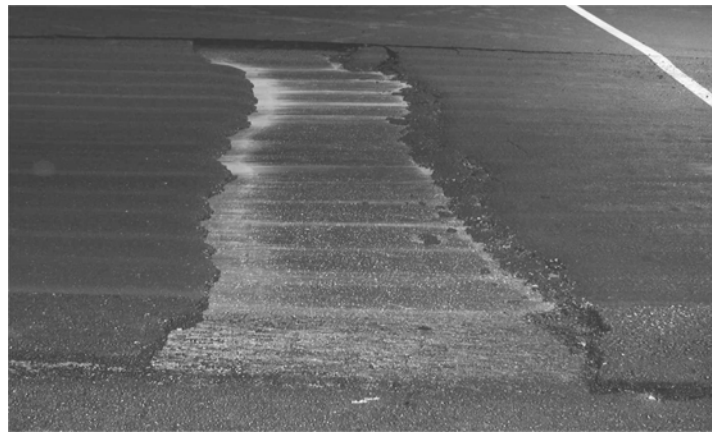
FIGURE 2-12. SEVERE SLIPPAGE CRACKING
