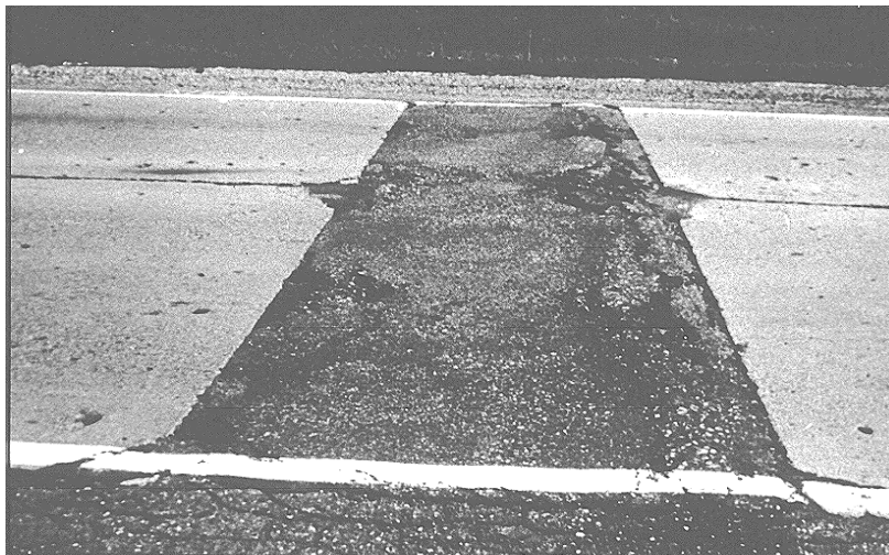
FIGURE 2-20. LARGE PATCH DISTRESS
