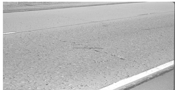
FIGURE 2-16. HIGH-SEVERITY TRANSVERSE CRACKING
