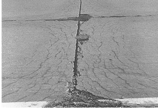
FIGURE 2-17. HIGH-SEVERITY D CRACKING
