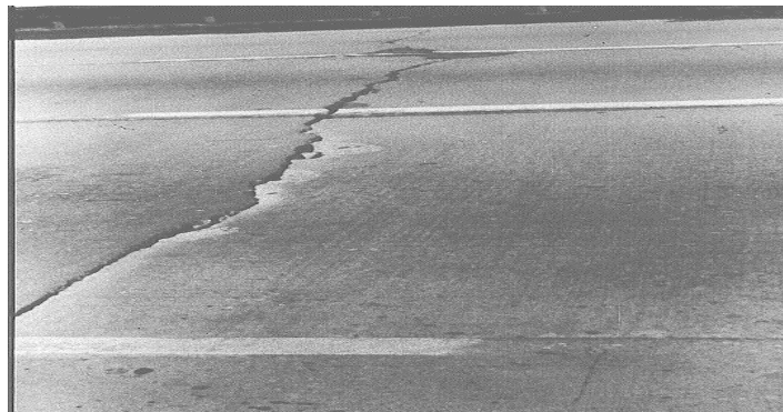
FIGURE 2-25. FAULTING OF TRANSVERSE CRACKS
