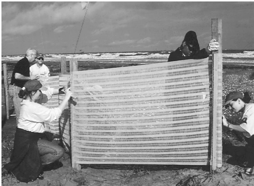
Six volunteers of a 150-member volunteer group attach webbing to a sand-trapping fence at Fourchon Beach along the Gulf of Mexico in Lafourche Parish. Volunteers constructed 5,000 feet of sand-trapping fence last April to help create new sand dunes on the beach, which has experienced dramatic erosion over the years. (NRCS photo)
