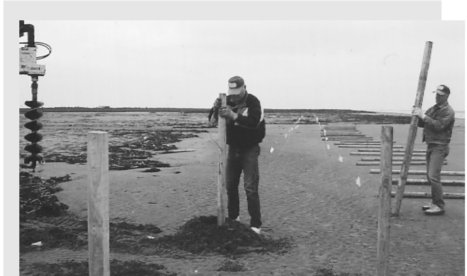
Don Gohmert (left) and Gary Fine insert treated timbers into the sand as part of the Fourchon sand-fencing effort. The group worked to construct 5,000 feet of sand-trapping fence at Fourchon Beach in south Louisiana along the Gulf of Mexico. (NRCS photo)
