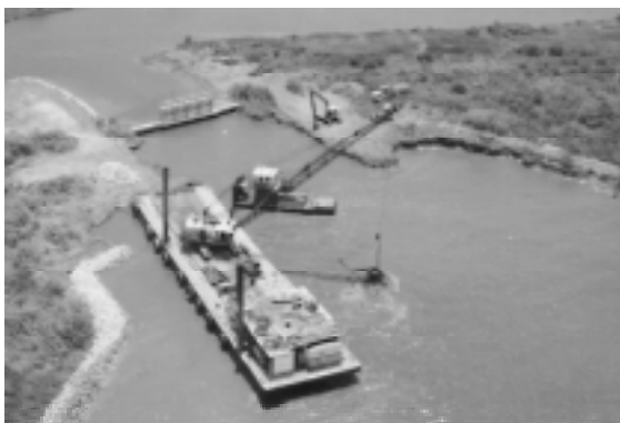
Construction contractors work from barge-mounted cranes to place rock around structures at Cameron-Creole. (ACOE photo)
