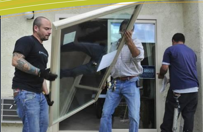
From Left: Andy Manzanera, Mark Hall, and Luis Cardenas install a double-pane patio window at Whispering Oaks Apartments in Ojai.
