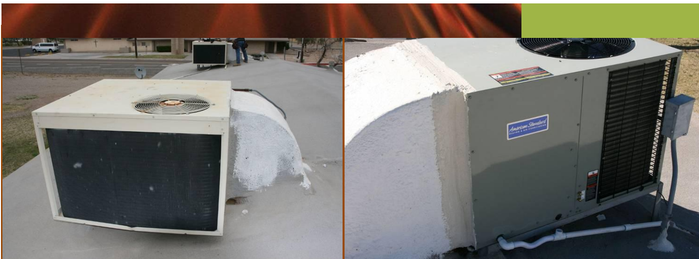
From Left: An old HVAC unit compared to a new unit installed at Needles public housing
