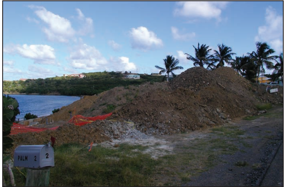
Figure 4.5. A large mound of dirt was excavated from a construction site located less than 100 m from the shoreline at Solitude Bay, St. Croix. Photo: C. Jeffrey.
