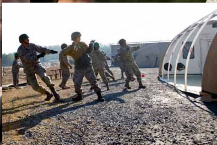
Lt. Col. Mark Vavra leads a team in pulling the top cover over a SSS structure during a Silver Flag exercise.
