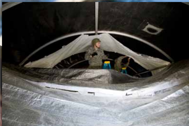
Tech. Sgt. Aaron Alden attaches the insulating liner of the SSS structure during the Silver Flag exercise.
