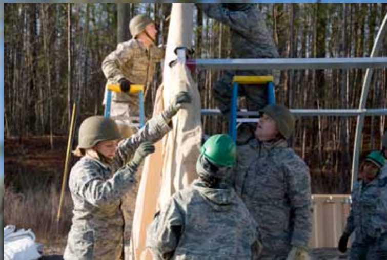
Tech. Sgt. Aaron Alden, Tech. Sgt. Thomas Bergl and Senior Airman Holly Kneisl work with other Air Force members to construct the front wall of a SSS (shade shelter system) structure during the Silver Flag exercise.
