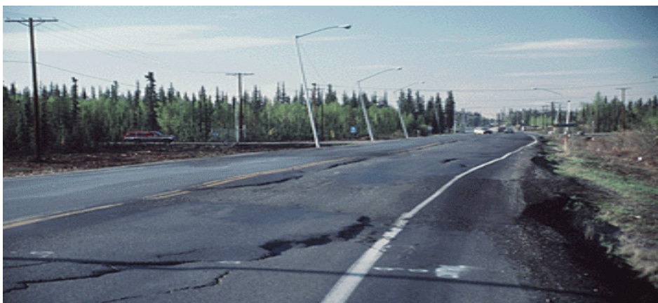
Figure 1. Photo of settlement and cracks on an Alaskan roadway due to warming of the permafrost foundation.
