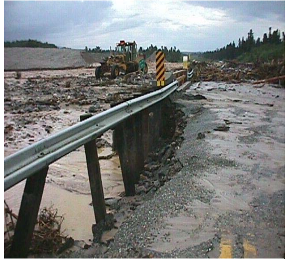
Figure 3. Photo of channel and bridge repairs after a flash flood at One Mile Creek.
