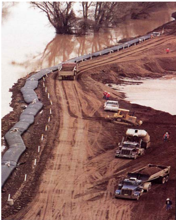
Figure 2. Photo of a levee breach in the Sutter Bypass. A warm winter storm in January 1997 caused this breach. A temporary bladder seen at left in the photo was used to protect the repair and prevent additional flooding from rising water levels in the bypass.
