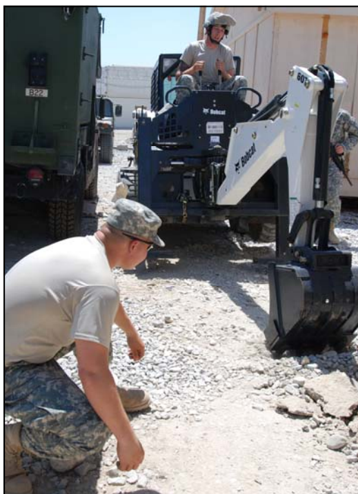
Pvt. Ben Williams (left), 76th Engineer Company based in Fort Knox, Ky., and attached to the 864th Engineer Battalion out of Fort Lewis, Wash., and Sgt. Christopher Masterson (right); Charlie Company, 173rd Special Troops Battalion, dig a trench to bury internet lines in the combat teams tactical operations center June 4 in Jalalabad Airfield. The airfield is under going significant changes over the next year to improve base structures.
